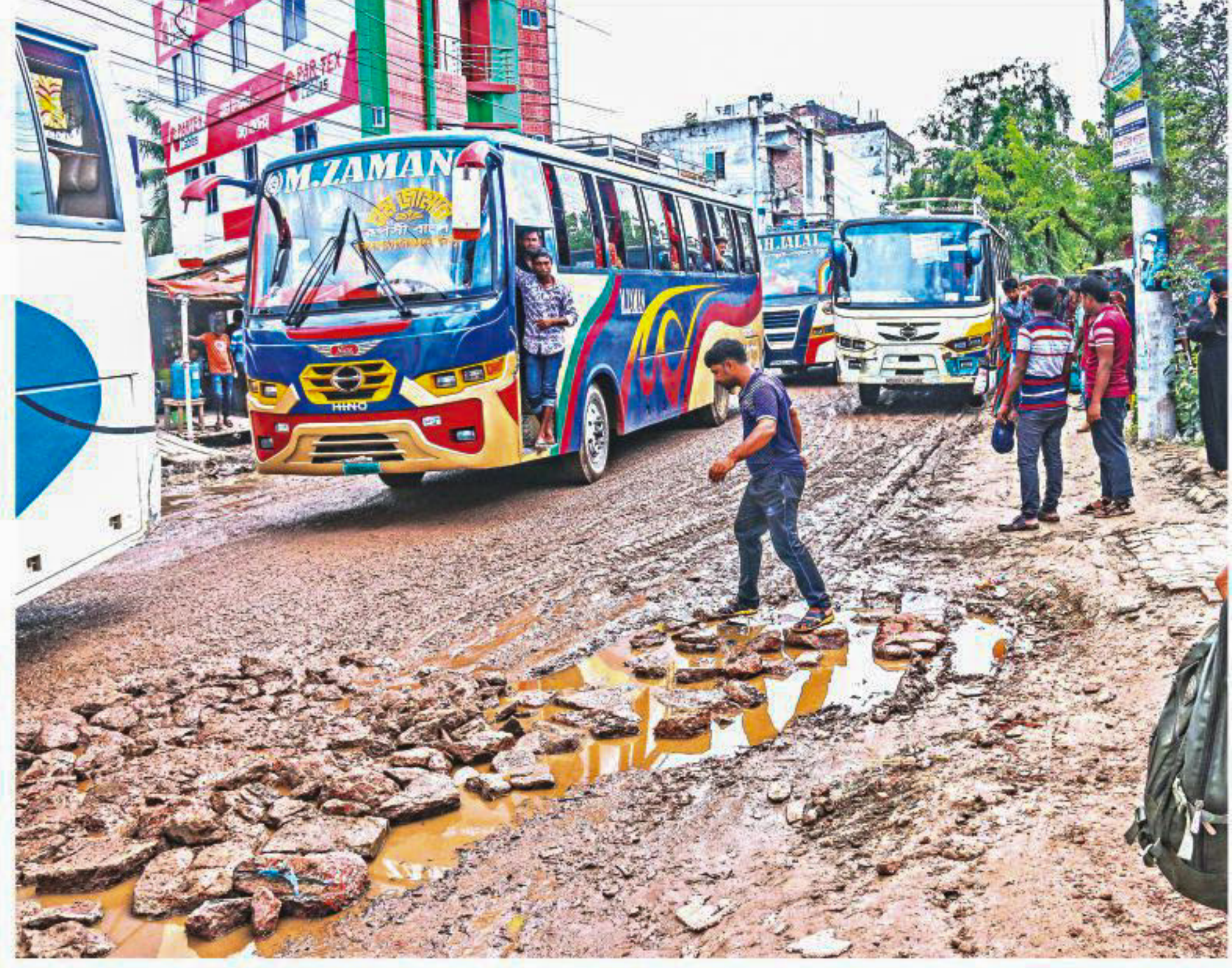
Buses to and from 18 districts -- including the capital -- enter and exit Khulna city through the road, that is neither suitable for vehicular movement, nor pedestrians'. PHOTO: STAR
