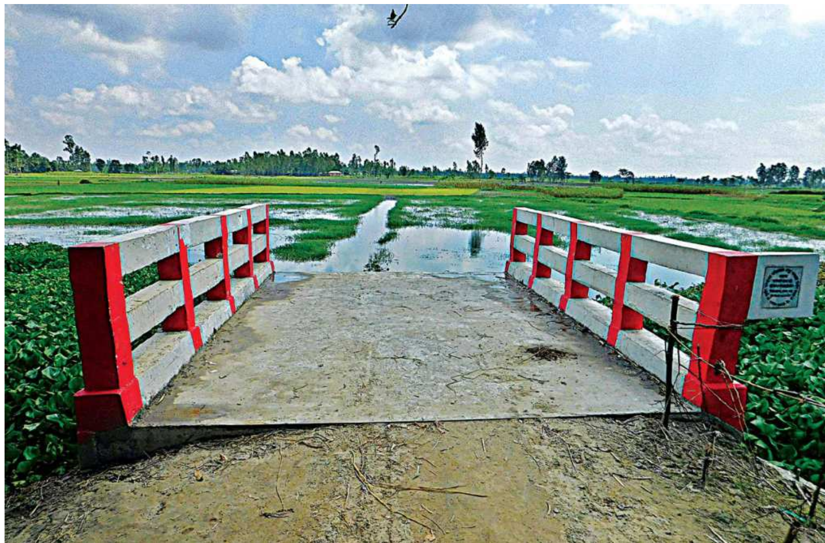
A BRIDGE TO NOWHERE: This small bridge without any approach road was built for Tk 14.85 lakh in Madhya Dighalkandi village of Bogura's Sonatola upazila. The photo was taken yesterday.
