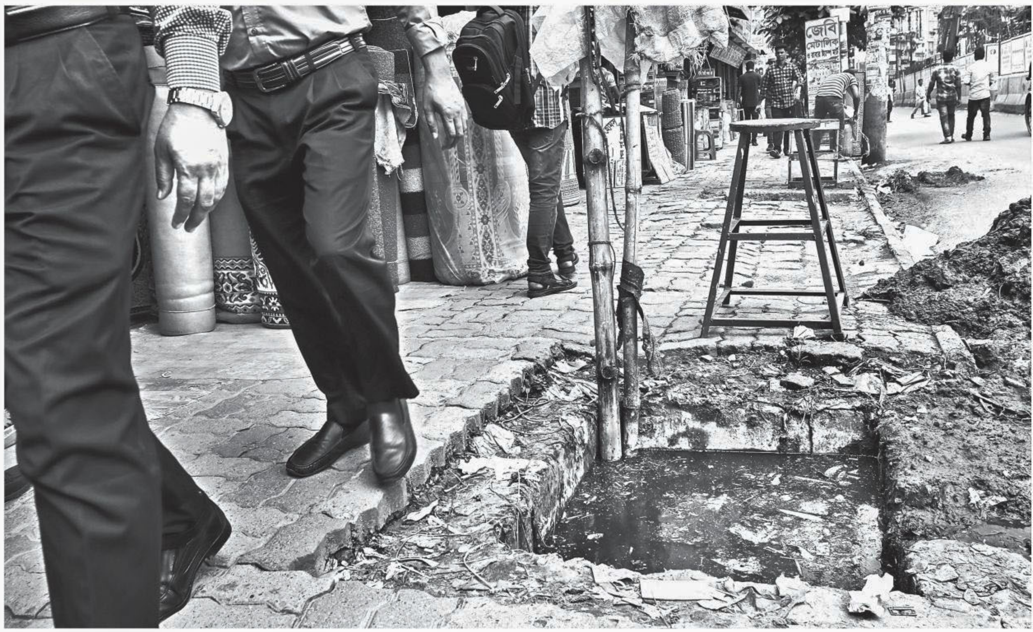
Pedestrians squeeze past a shop and a gaping drain on a footpath in Purana Paltan in the capital. The only warning about the drain is two bamboo poles sticking out of it, although such holes should be covered. The photo was taken yesterday.
