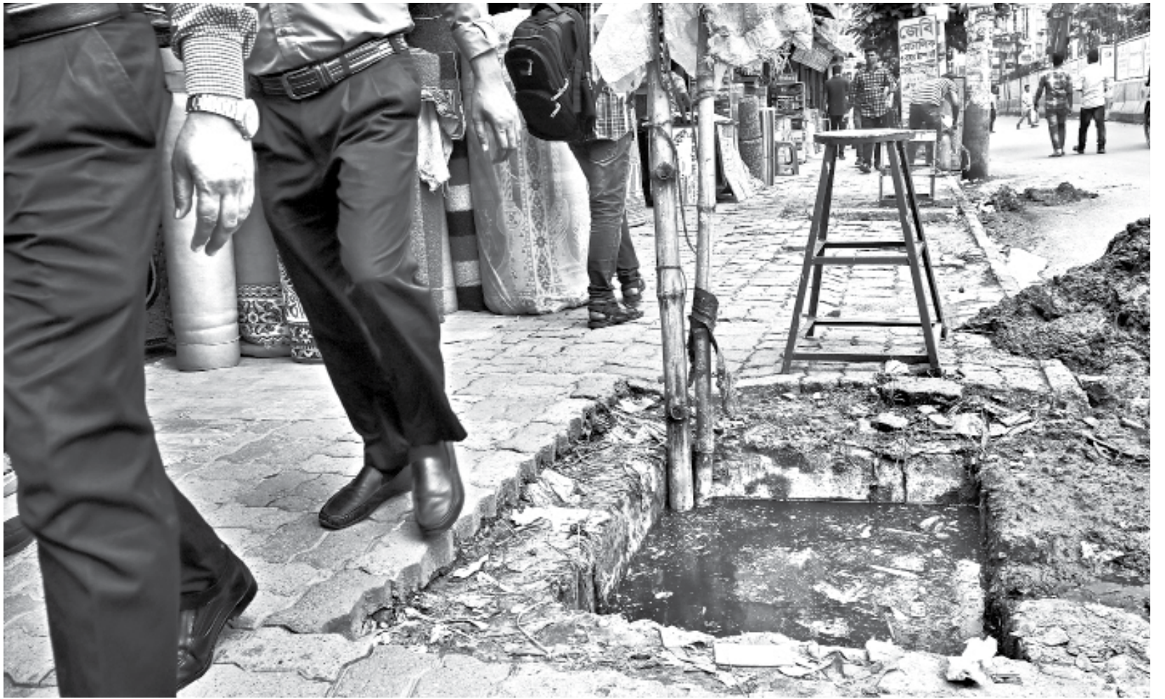
Pedestrians squeeze passed a shop and a gaping drain on a footpath in Purana Paltan in the capital. The only warning of the drain is two bamboo poles sticking out of it, although such holes should be covered. The photo was taken yesterday.
