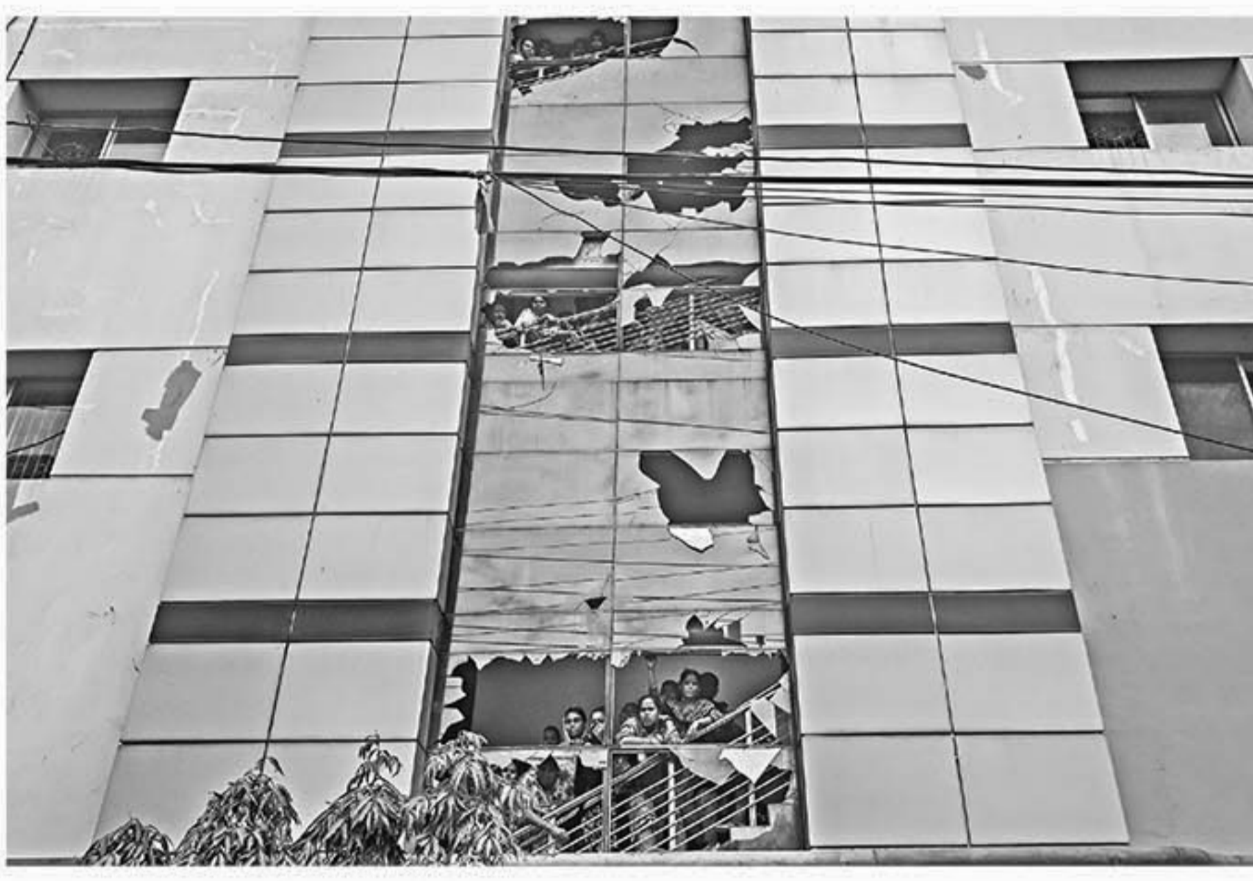
Broken windows of the RMG factories in the port city. PHOTO: STAR
