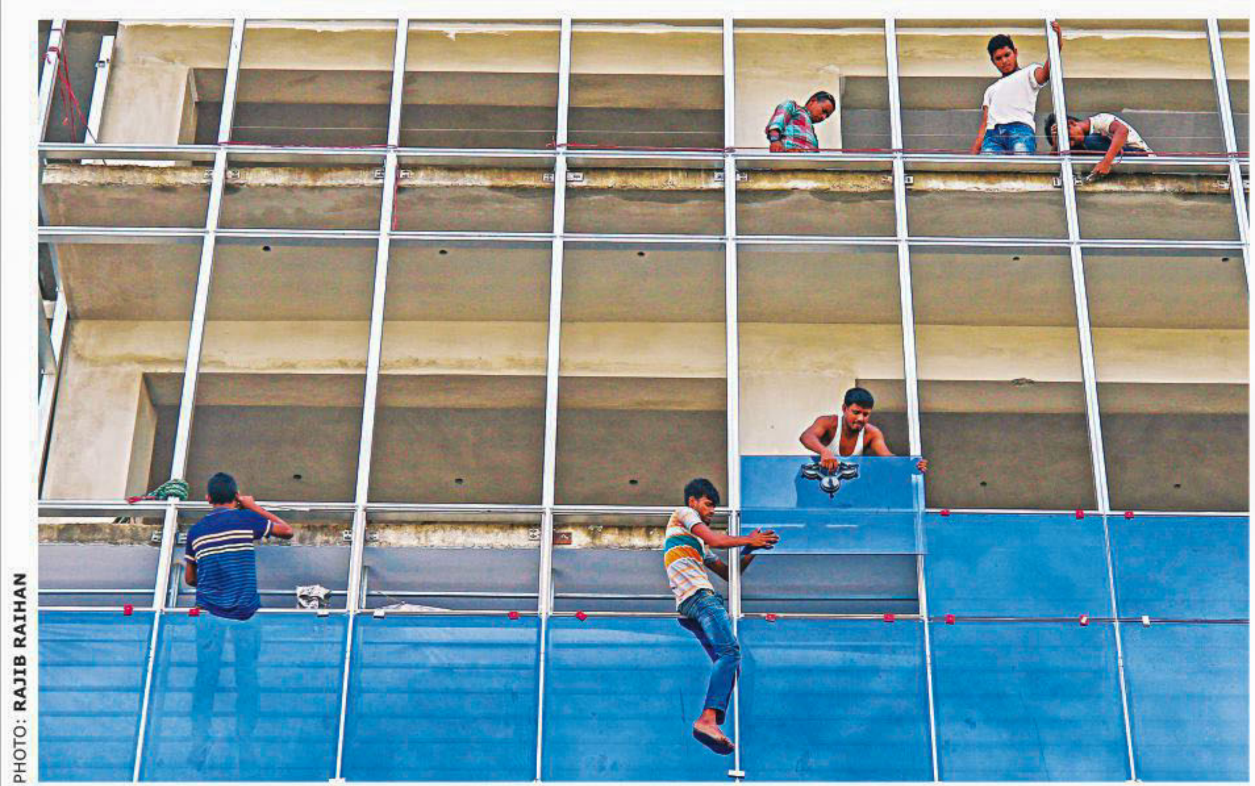
Workers install glass panels on a high-rise in Chattogram while sitting and leaning precariously on the frames without any form of harness. The photo was taken yesterday at Wasa intersection in Dampara.
