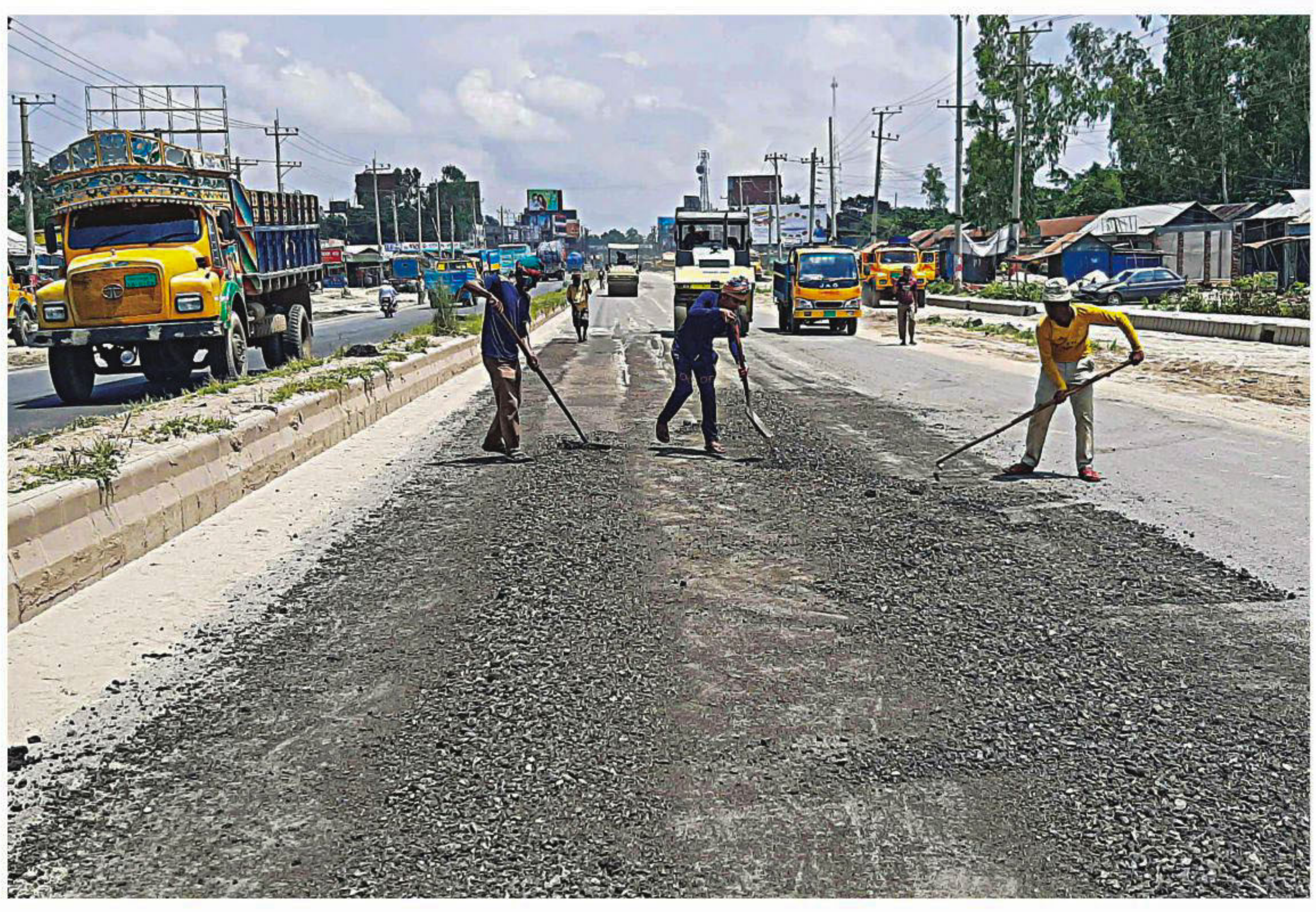
Workers repair the grooves created by the continuous plying of heavy vehicles on Dhaka-Tangail highway at Elenga. Eid holidaymakers fear there would be a lot of traffic jams and bottlenecks on this highway during the Eid rush. PHOTO: MIRZA SHAKIL
