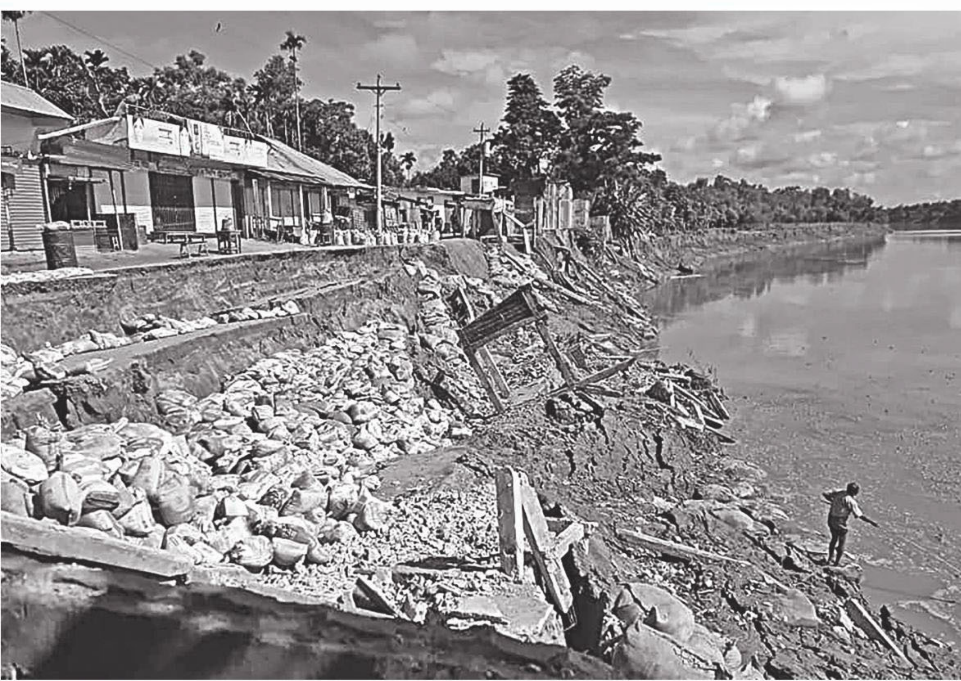
A large section of flood control embankment alongside the Manu river in Moulvibazar's Kulaura upazila was eroded by the river this Thursday. Except for hastily dumping some sandbags, Water Development Board, however, took no effective step to protect it.
