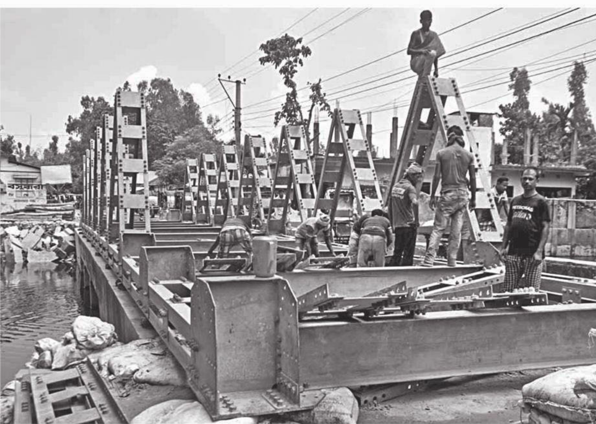
Roads and Highways Department is setting up a Bailey bridge replacing a concrete bridge that tilted due to the impact of surging floodwater on Gaibandha-Sundarganj highway at Kadomertola in Gaibandha town. PHOTO: STAR
