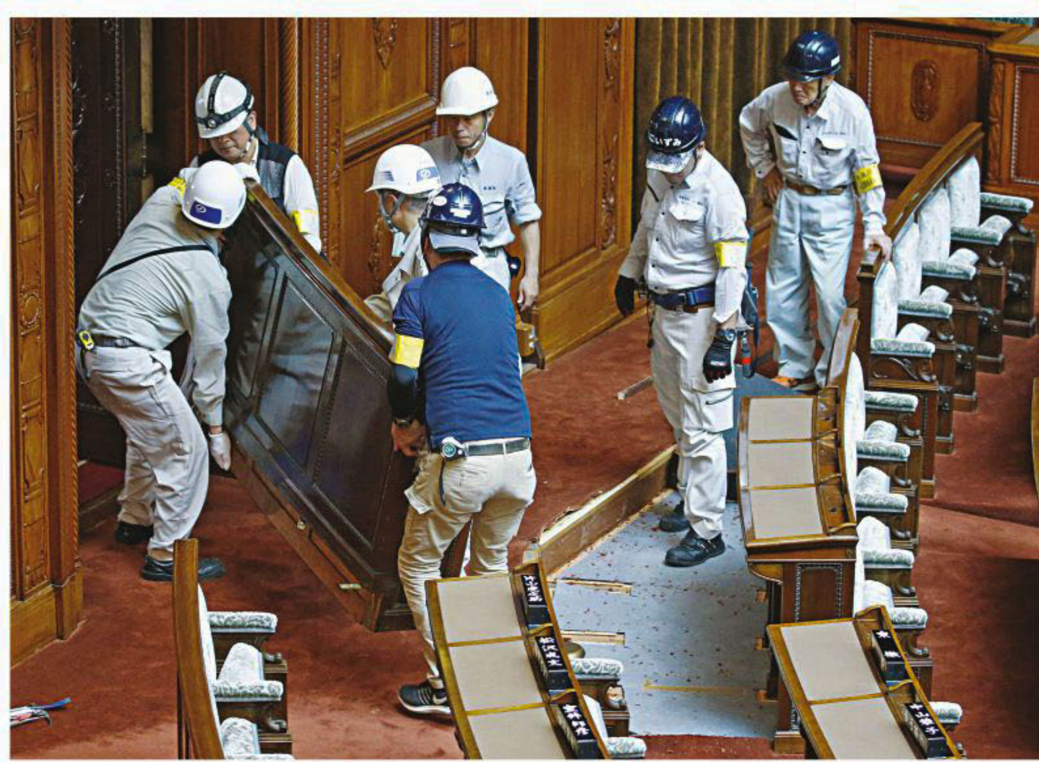
Workers start the renovation to prepare a barrier-free area for two newly elected lawmakers with severe physical disabilities at the upper house of parliament hall in Tokyo, Japan. The photo was taken on Sunday.
