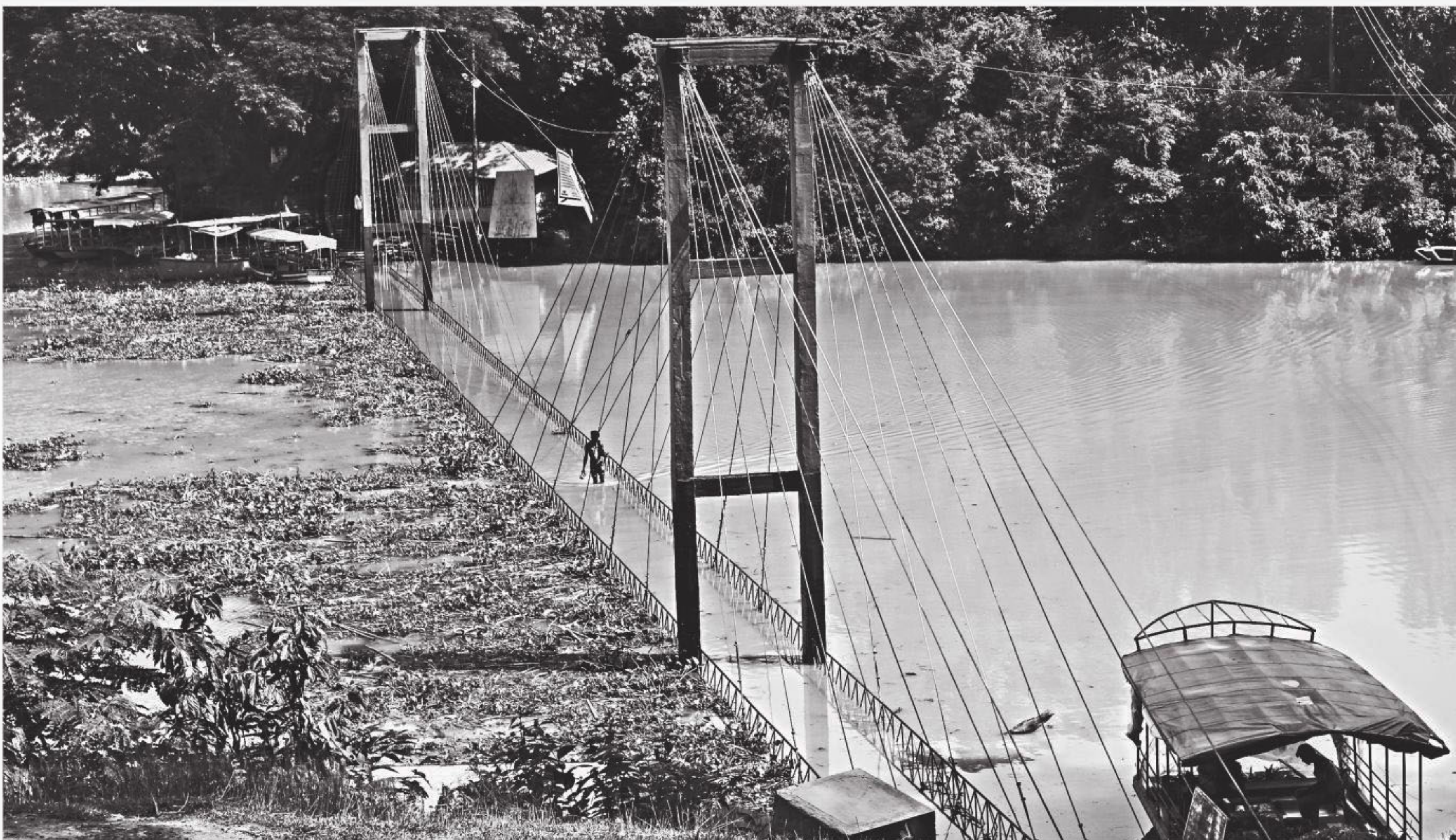
Rainwater submerges the hanging bridge over Kaptai Lake in Rangamati, compelling the authorities to suspend movement of people on the bridge.
