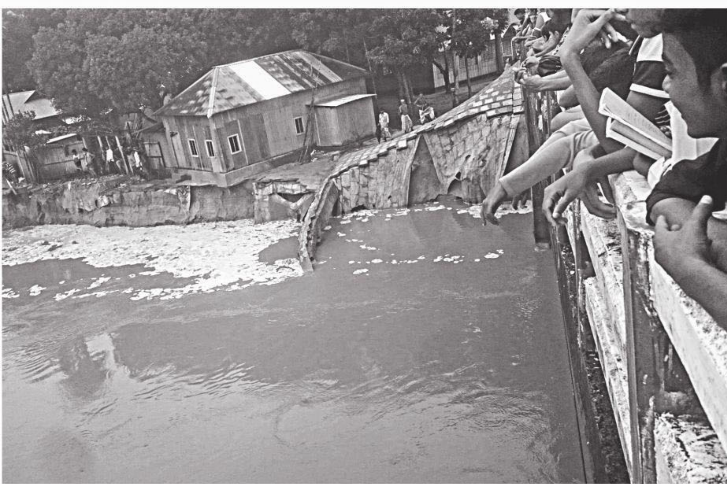
Concrete blocks on the west side of the guide embankment of a newly constructed bridge on the Pungli river in Borobasalia area of Tangail Sadar upazila collapsed on Saturday due to heavy rain, leaving the bridge and nearby dwellings at erosion risk.
