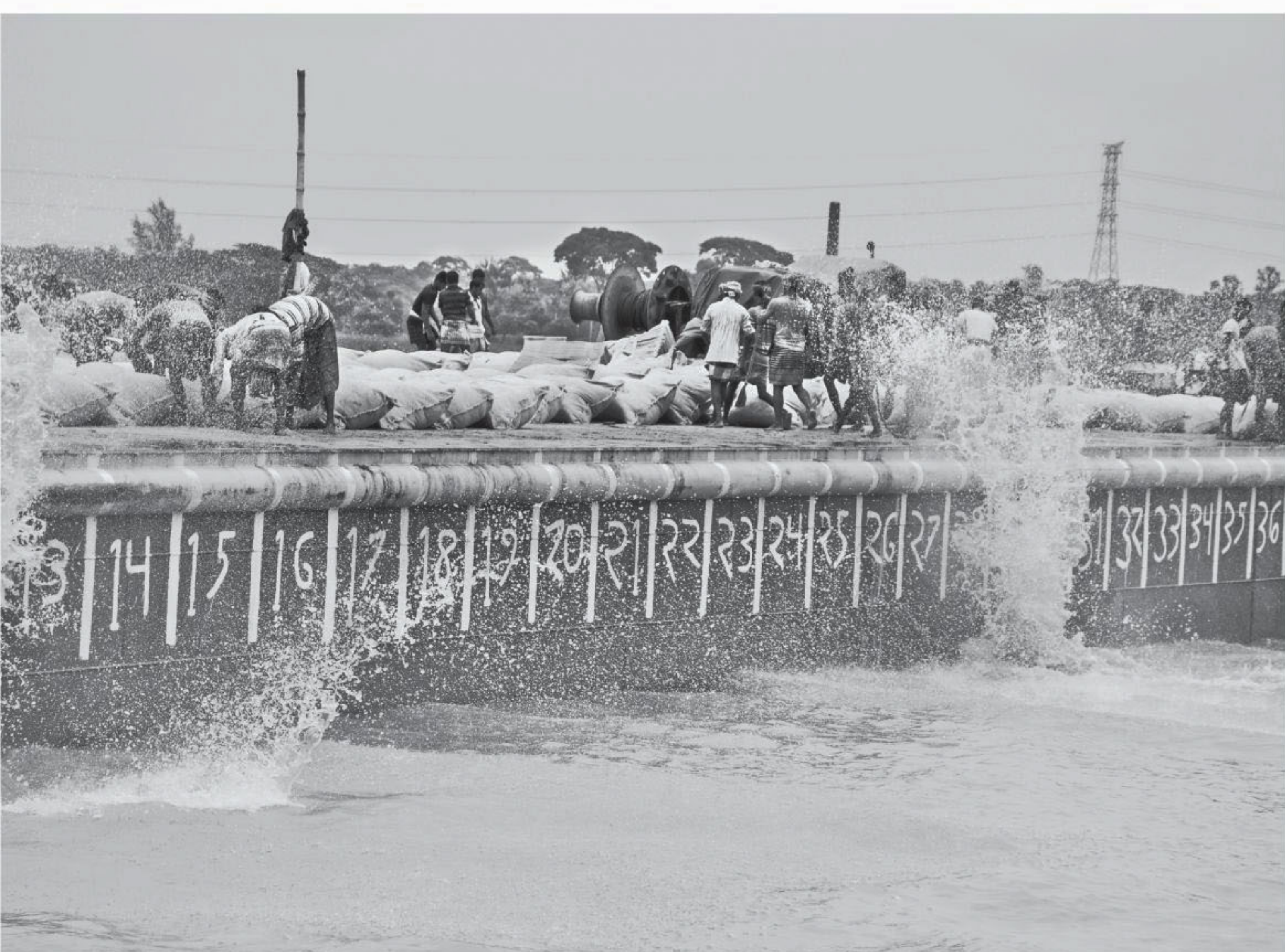
Workers throw in sand-filled bags into the Kirtankhola river, in an effort by Bangladesh Water Development Board to prevent erosion on the river. The photo was taken from Beltola area of Barishal city earlier this week. PHOTO: TITU DAS
