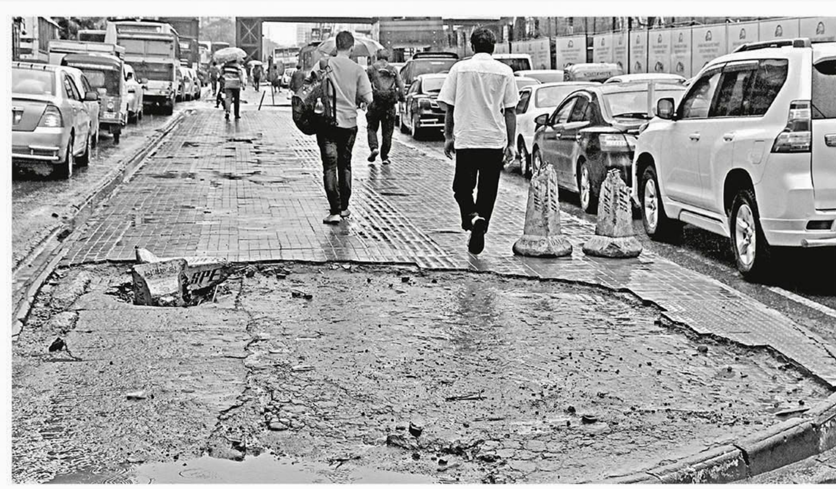
The footpath on the capital's Kazi Nazrul Islam Avenue is in a dilapidated state with holes covered by concrete posts and puddles formed by rain. The photo was taken yesterday.
