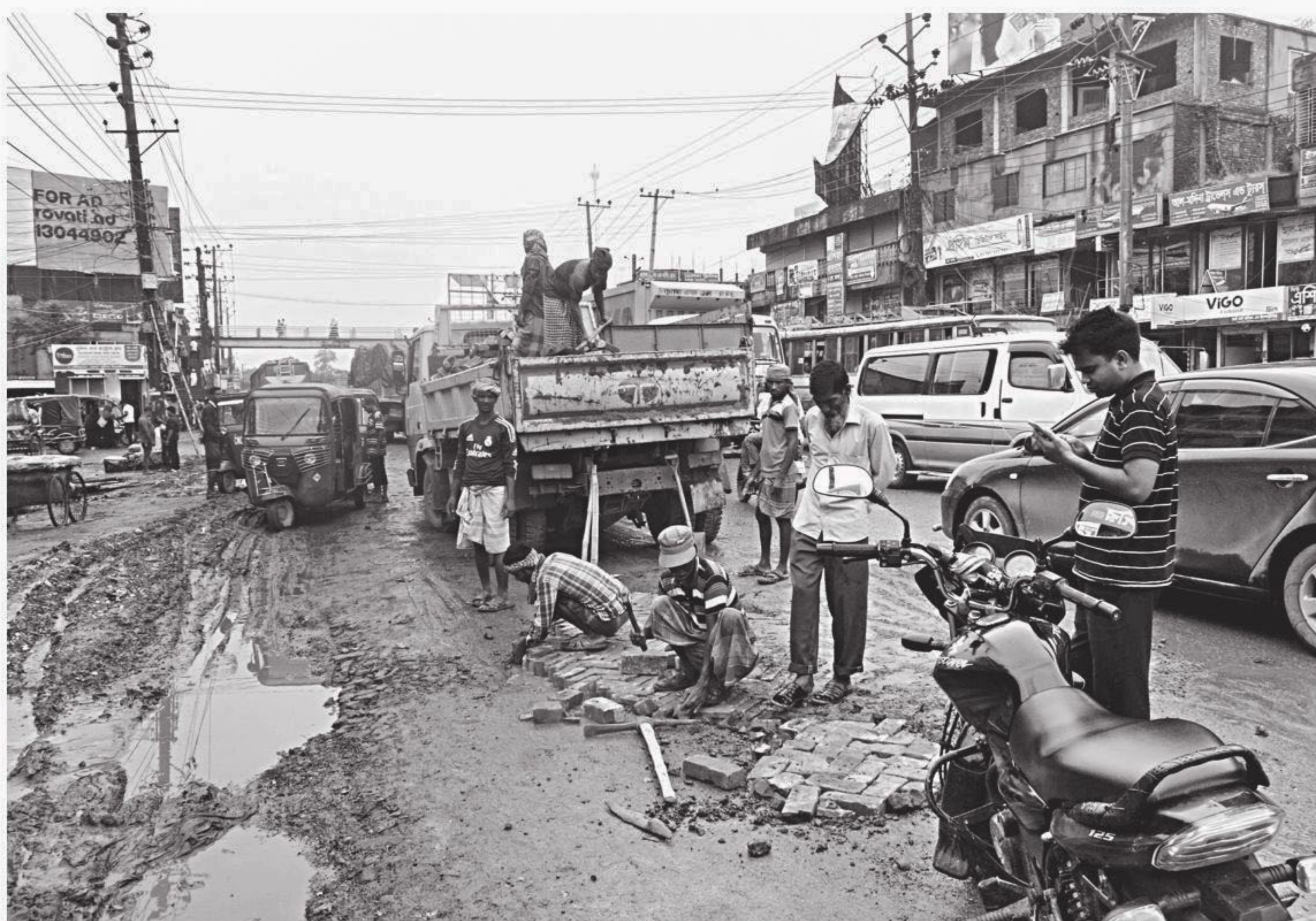
Workers, employed by the Roads and Highways Department in Tangail, are seen repairing the busy road in Elenga Bus Stand area in Tangail's Kalihati upazila yesterday. The important spot on Dhaka-Tangail highway has been badly damaged due to heavy rain in the last three days.
