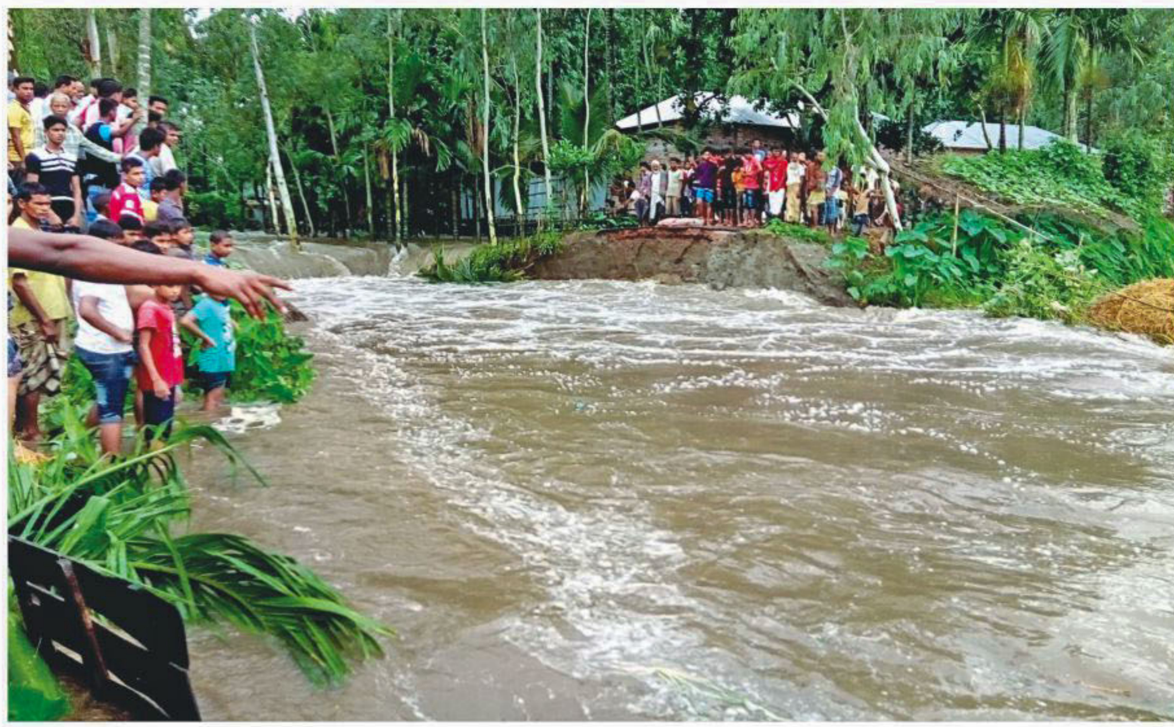
People watch as water from the swollen Teesta river gushing into their neighbourhood in Gaddimari area of Lalmonirhat's Hatibandha upazila after a part of the protection embankment collapsed yesterday afternoon.
