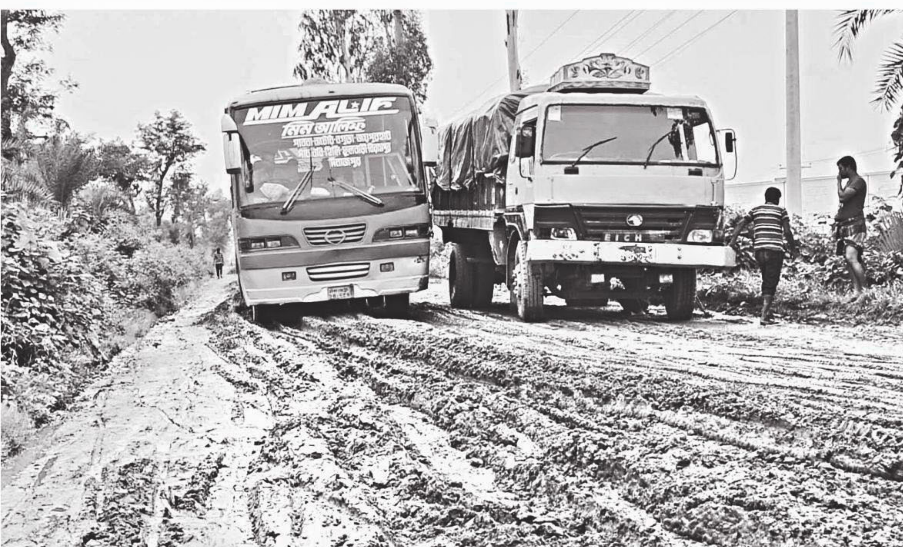
A large section of Joypurhat-Bogura highway lies in an awful condition, posing serious risk of accident for vehicles plying the important road. The photo was taken from Kalai Bazar area in Joypurhat's Kalai upazila on Wednesday.
