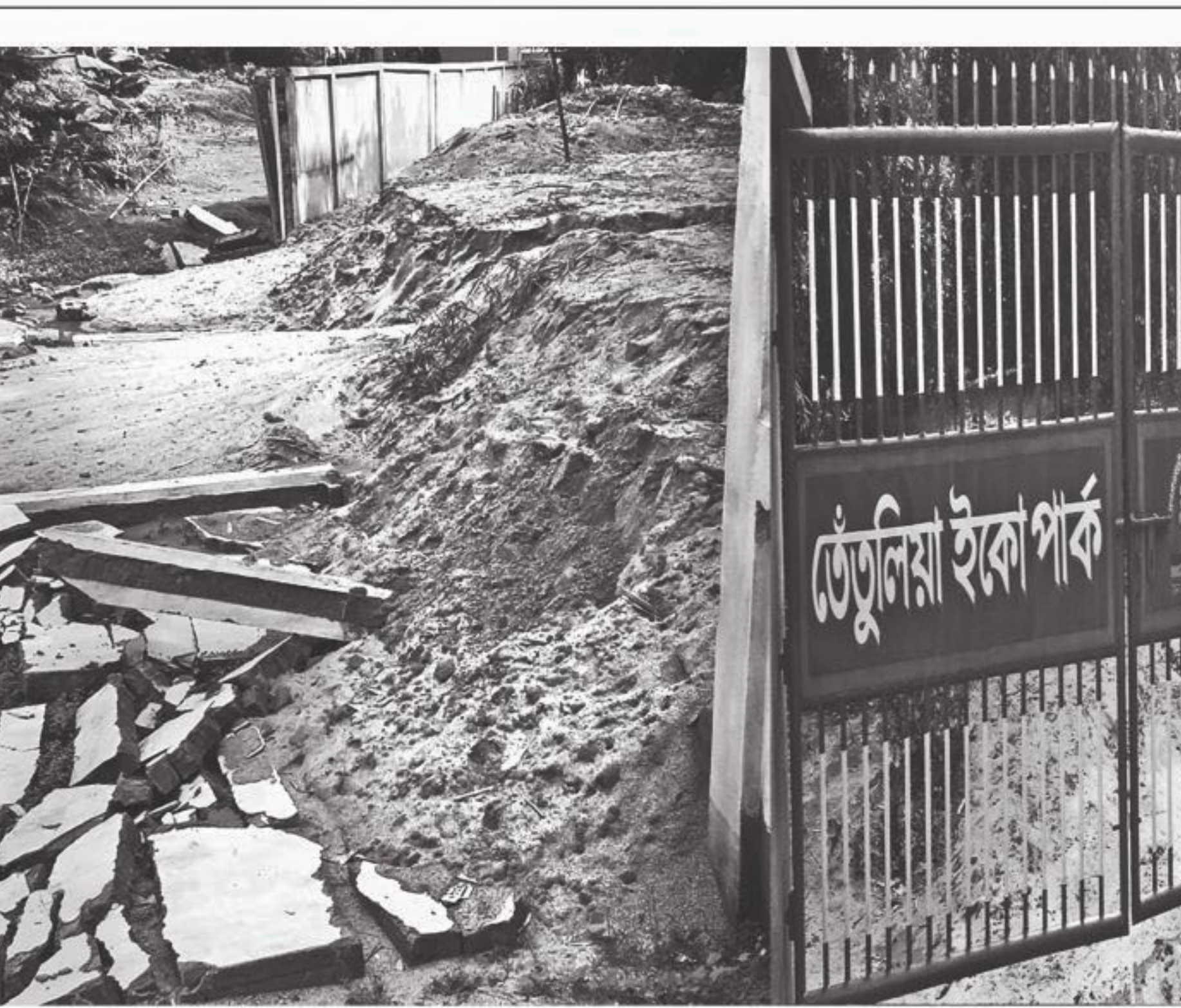
Chunks of concrete lie scattered as a part of the boundary wall of Tentulia Eco Park collapsed on July 5.
