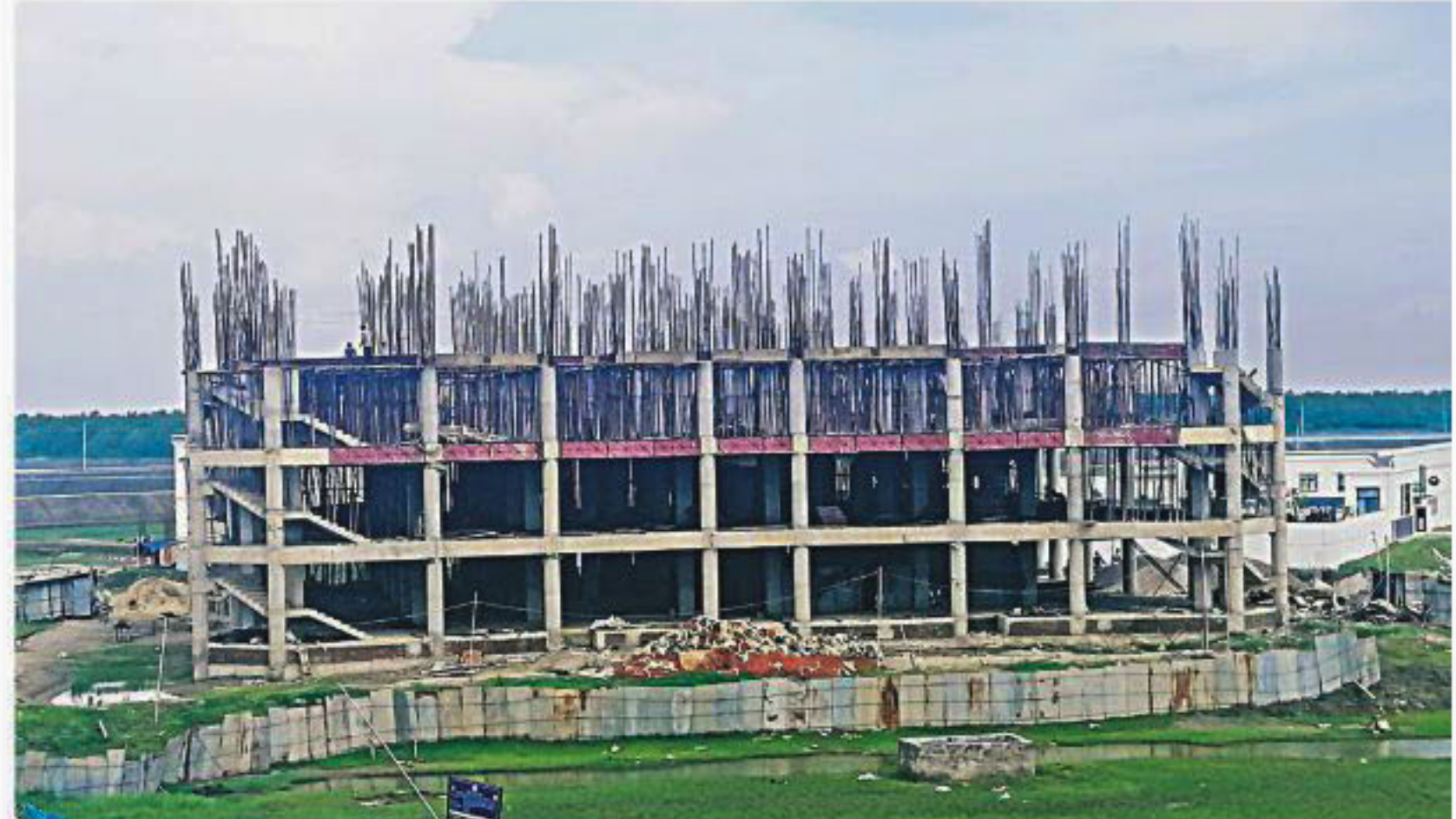
Construction work is going on at a factory inside Mirsarai Economic Zone in Chattogram.
