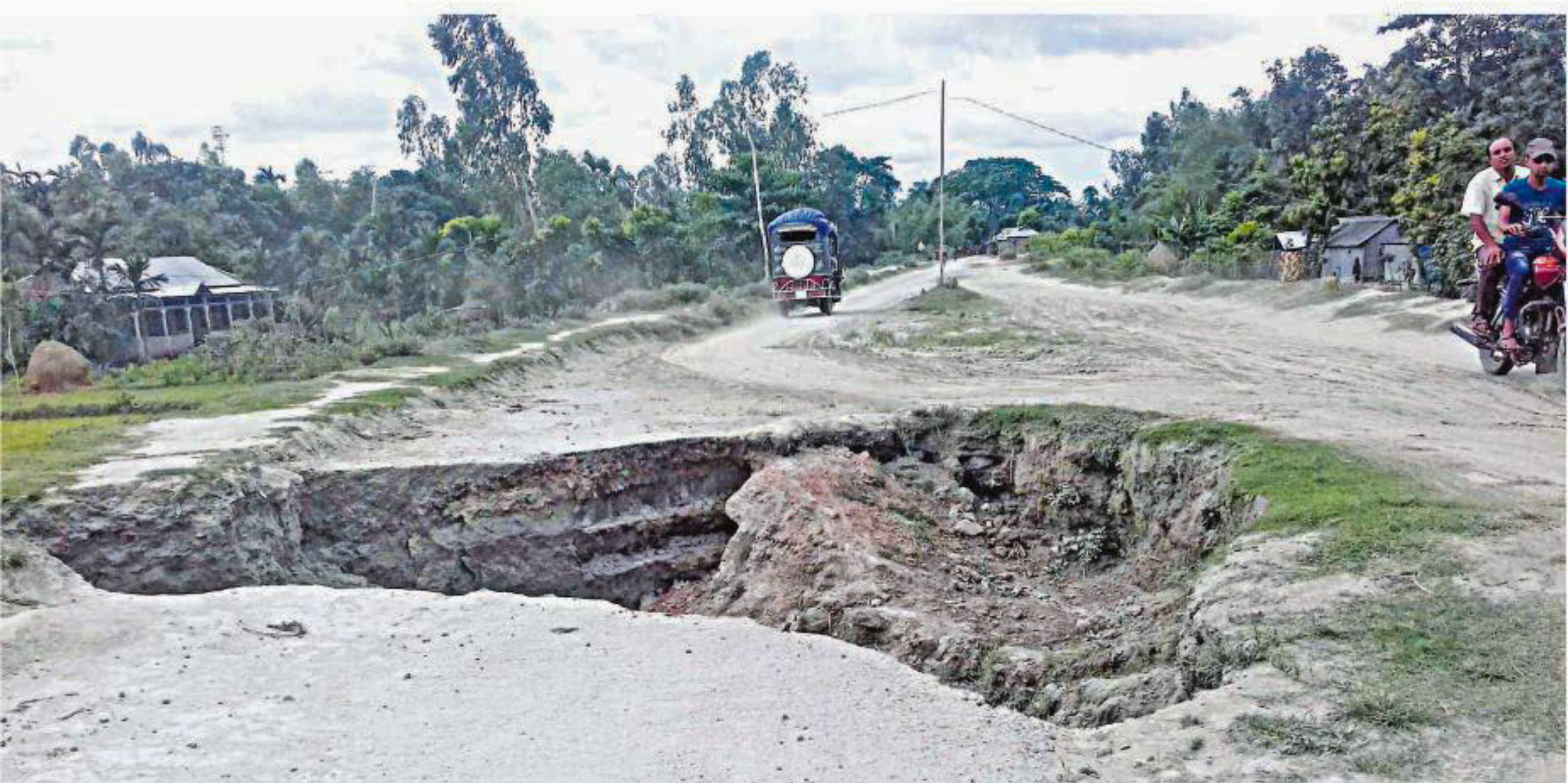
Large cracks, like this one at Dhumaitari of Sundarganj upazila of Gaibandha, have developed on Sundarganj-Kamarjani flood control embankment-cum-road on the western bank of the Brahmaputra river amid heavy rain during the last one month, posing threat of erosion in a large area.
