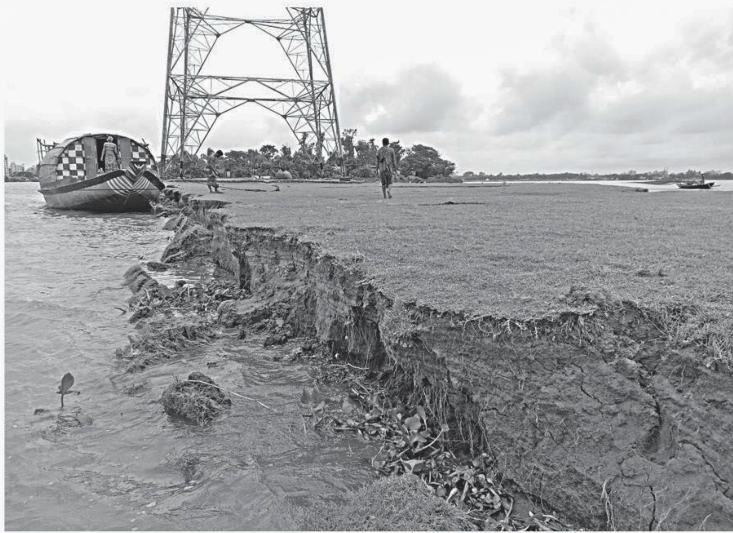
The Ashuganj-Shambhuganj National Power Grid is under threat as the Meghna is devouring Charsonarampur in Ashuganj of Brahmanbaria. The photo was taken recently.
