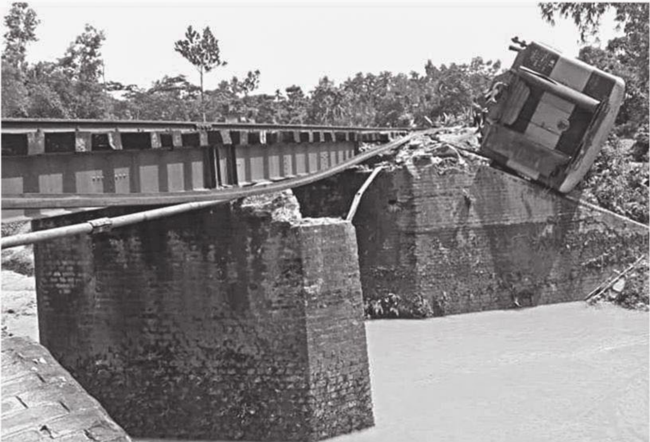
The spot of train accident near Baramchal railway station in Kulaura upazila of Moulvibazar on June 23. Right, loose and missing nuts and bolts on a rail track in Srimangal area in Moulvibazar shows awful condition of the track.
