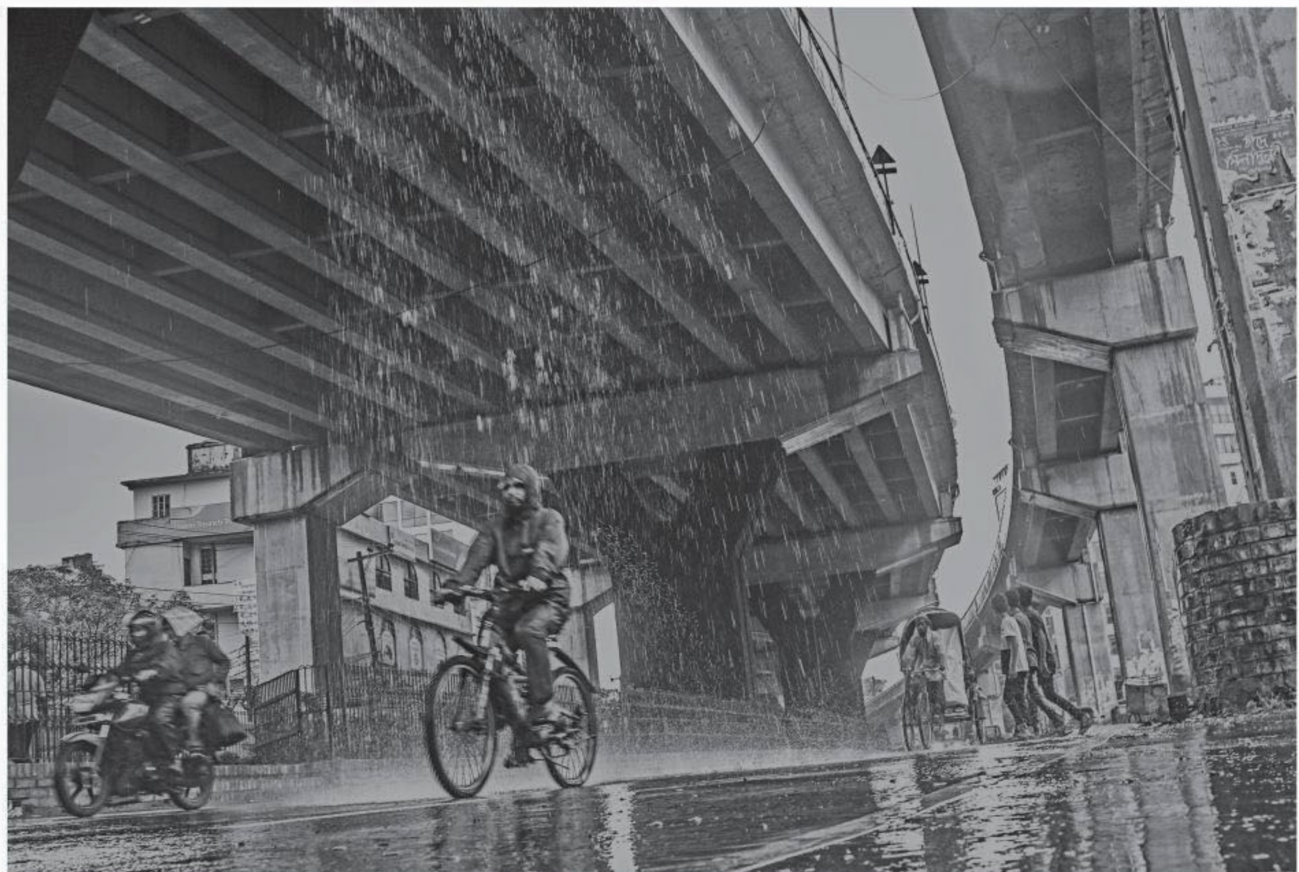
Water clogged on Akhtaruzzaman Flyover fall through its ceiling as the pipes meant for removing rainwater got damaged. The authorities concerned are so far indifferent to the situation. The photo was taken in Chattogram city's GEC area yesterday.
