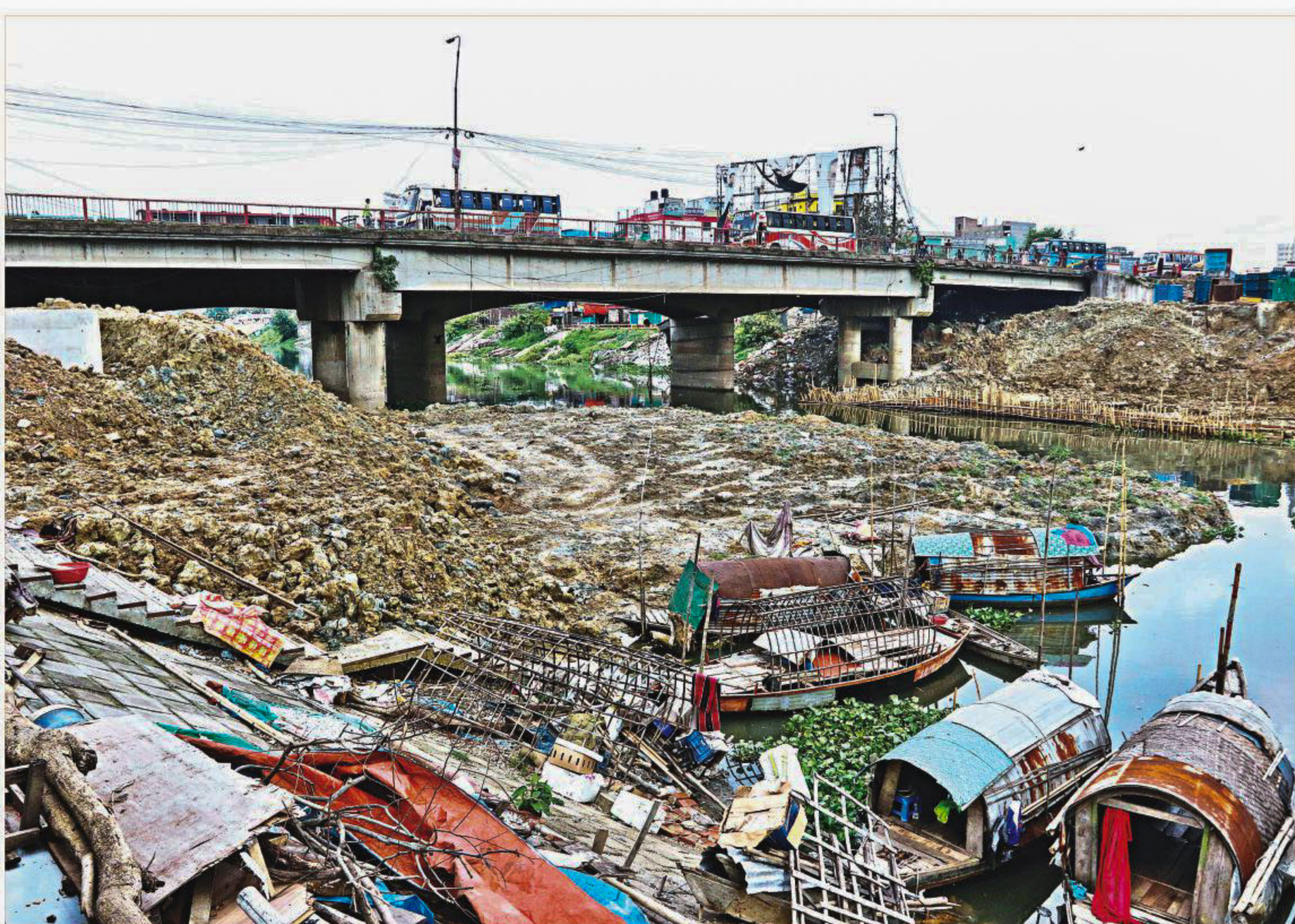
The Turag is almost completely choked near the Tongi-Abdullahpur Bridge at the northern edge of the capital as piling work for a new bridge is going on. The photo was taken last month. PHOTO: ANISUR RAHMAN
