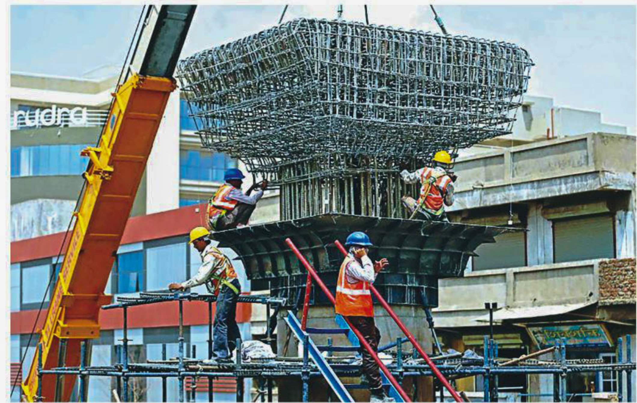
Labourers work at the site of an under-construction metro railway flyover in Ahmedabad, India.
