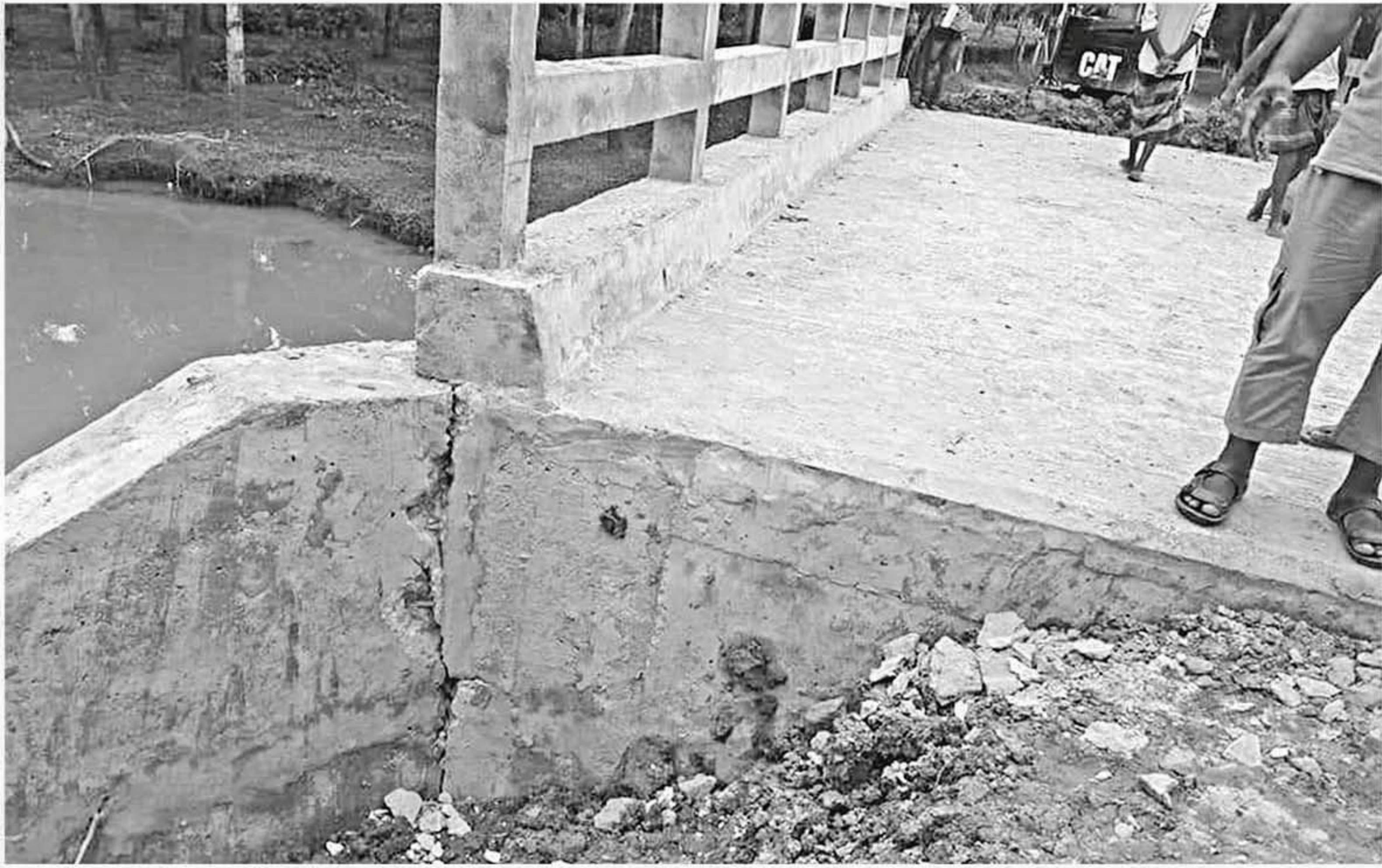
Even before handing over, large cracks have developed on this newly reconstructed bridge on Akhali canal in Moulvibazar's Kulaura upazila.
