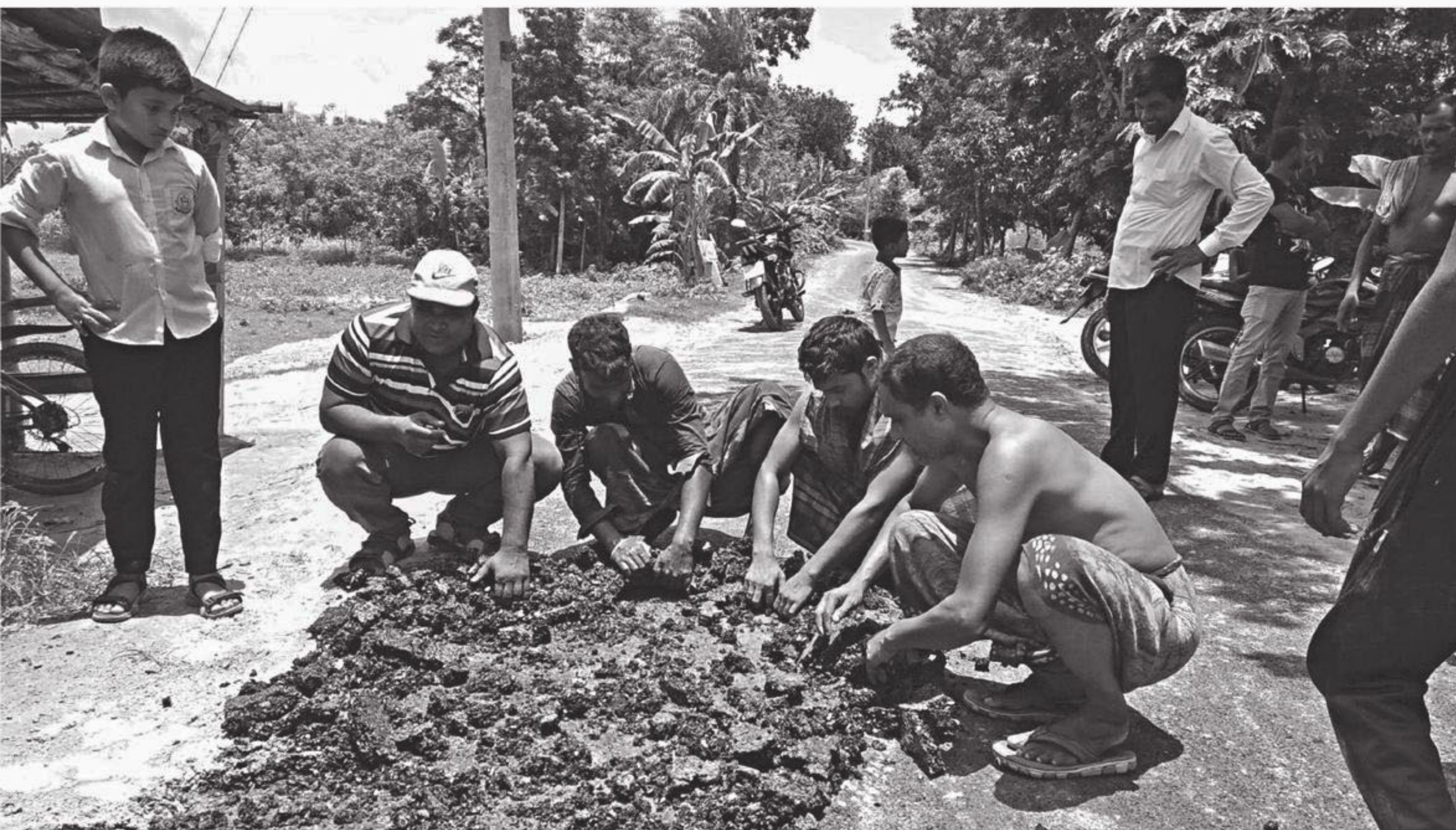
Locals in Dharmadah village under Kumarkhali upazila demonstrate how asphalt paving of the newly built road in the village is coming off without using any tools. The photo was taken recently.
