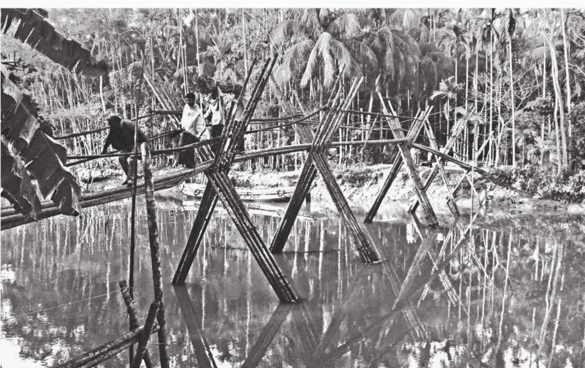
People have to cross amid risk the rickety bamboo bridge at Singor-Chandipur village in Morrelganj upazila of Bagerhat as the authorities concerned have not taken any initiative after a concrete bridge at the spot collapsed 12 years ago.
