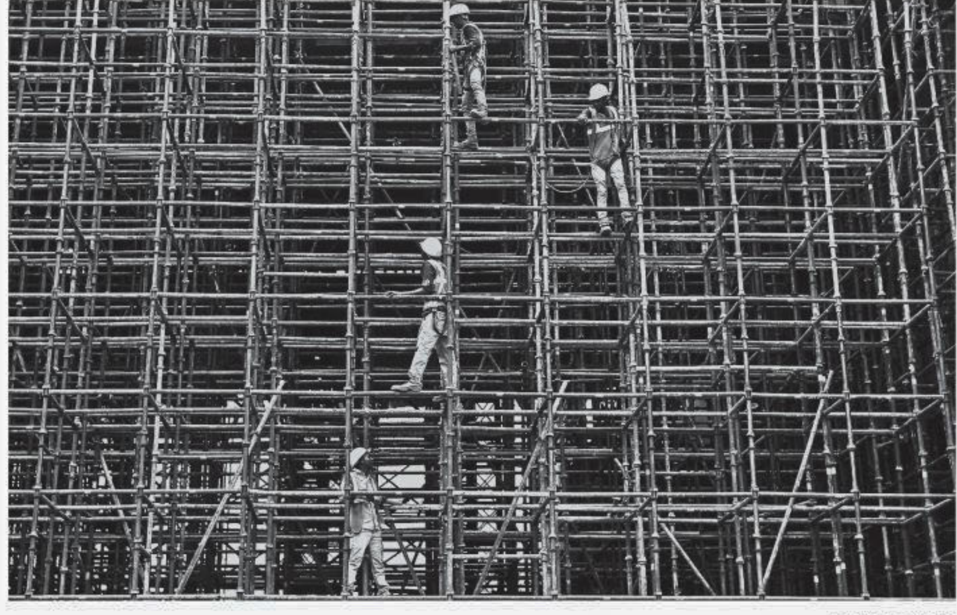
Labourers work at a construction site of a metro rail station in Kolkata.
