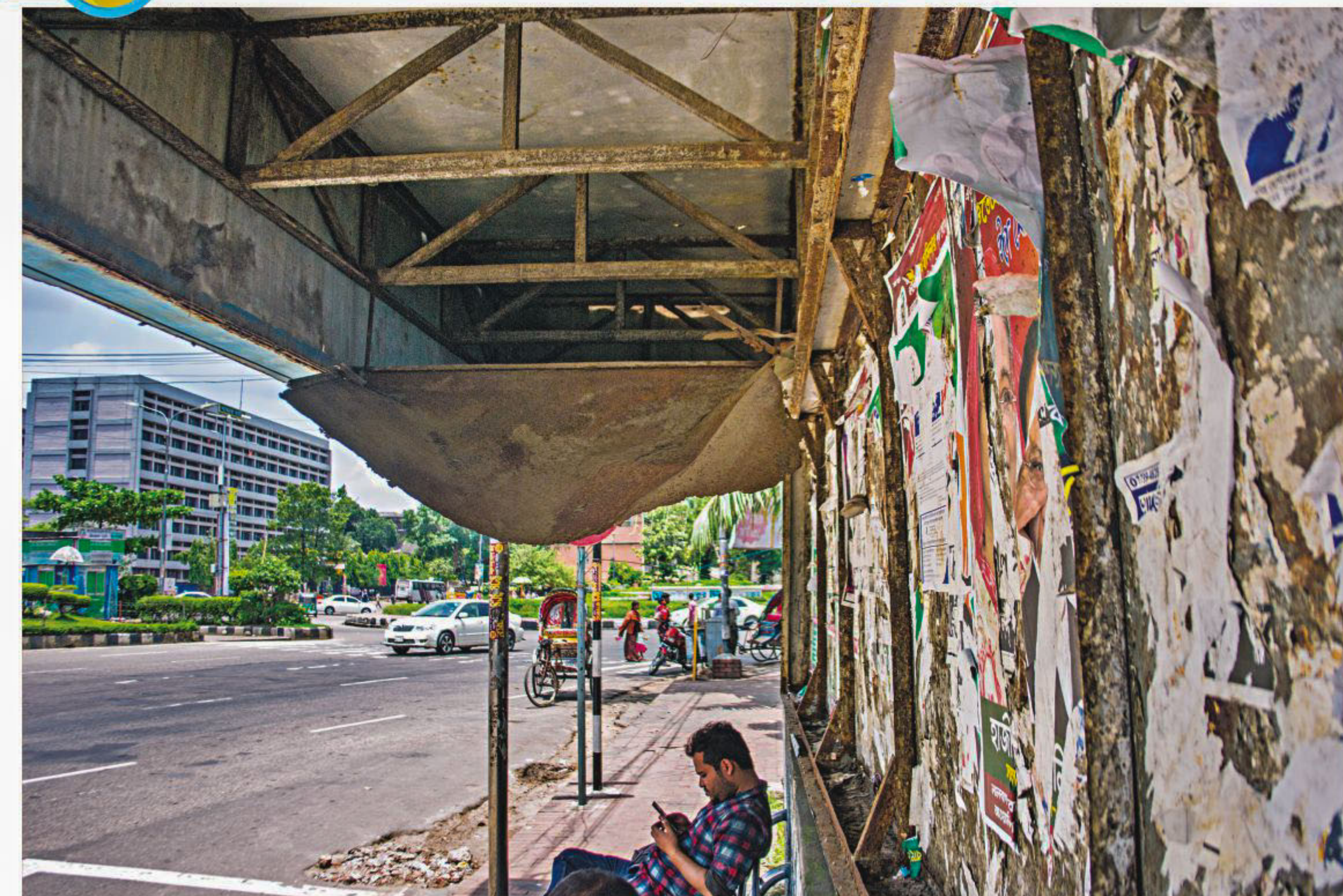
Busy on phone, a man sits at a place which once probably was a bus stop while the last remaining metal panel of this ramshackle passenger shed hangs precariously right above him. The shed is supposed to protect commuters from heat and rain. Instead, it has become risky for people. The photo was taken on Manik Mia Avenue recently.
