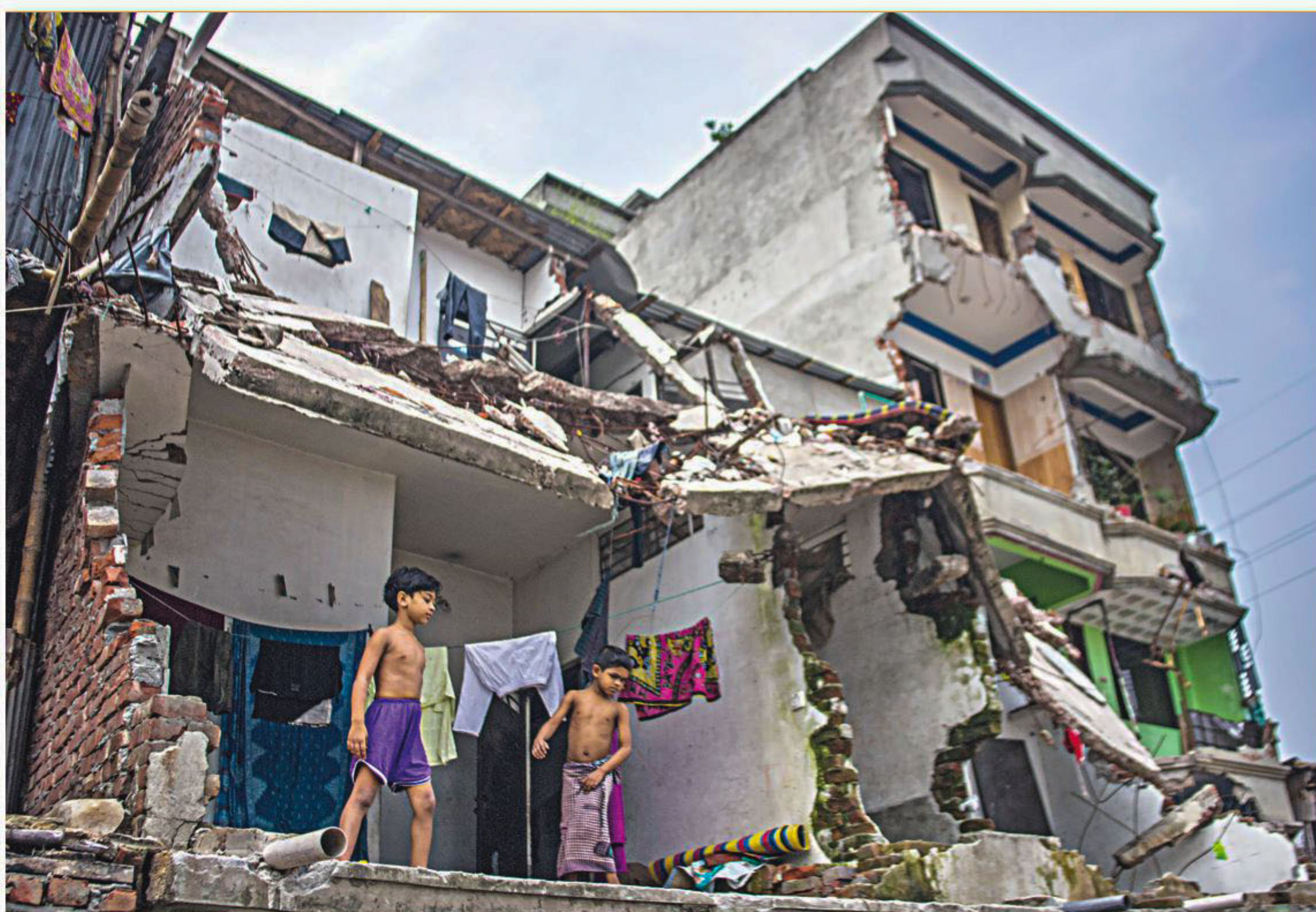
The BIWTA had knocked down illegal parts of these buildings on the Buriganga in the city's Islambagh area over three months ago, but they are still occupied by people and that too without any repair. Such use of the buildings might put the occupants in harm's way. The photo was taken yesterday.
