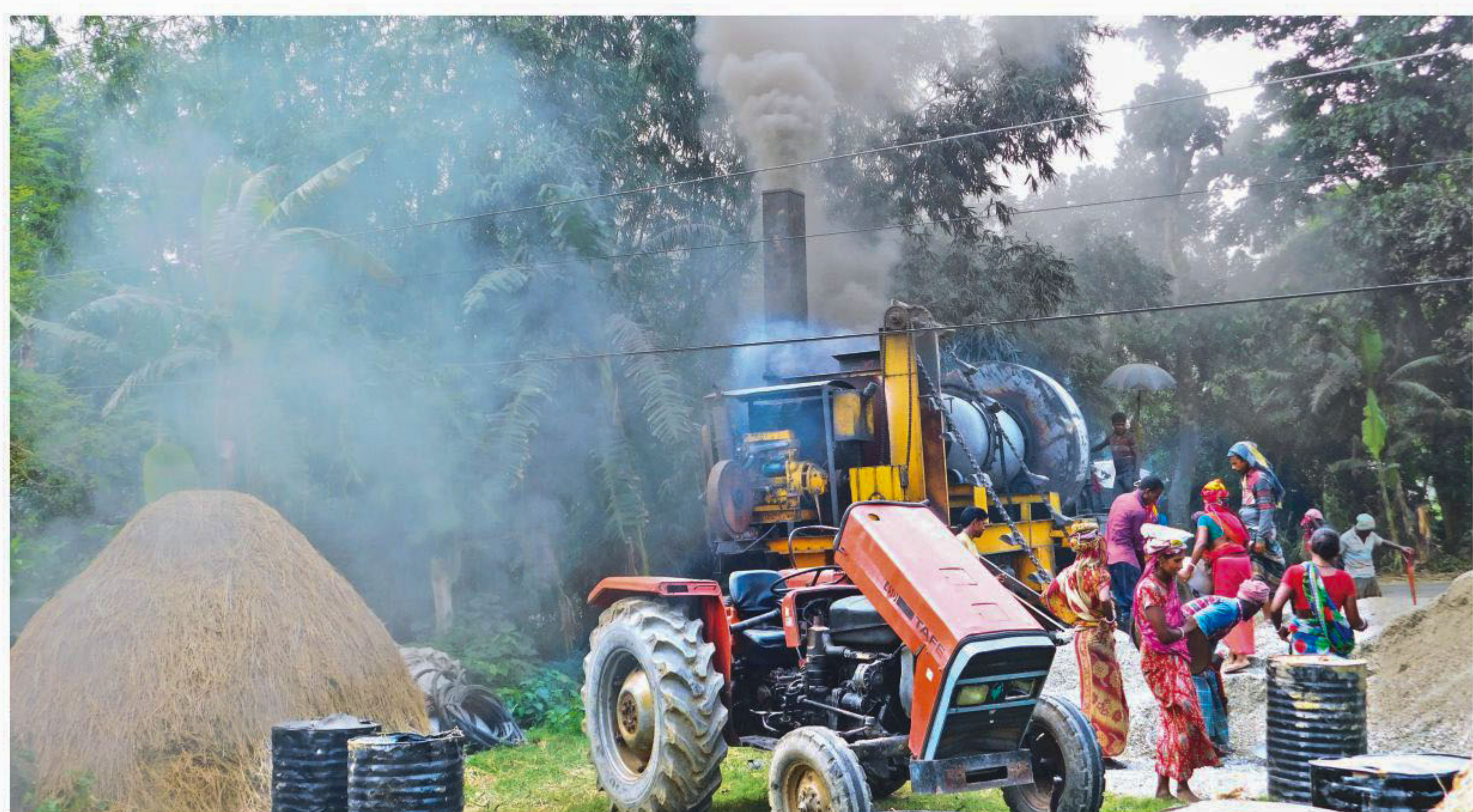
An asphalt-mixer spews out a cloud of smoke during road repair works in Nepaltali village in Bogura's Gabtoli upazila. The use of such high polluting machines is prohibited in residential areas by the Department of Environment. Additionally, the workers appear to not have been given any protective masks, putting them at risk of contracting respiratory diseases.
