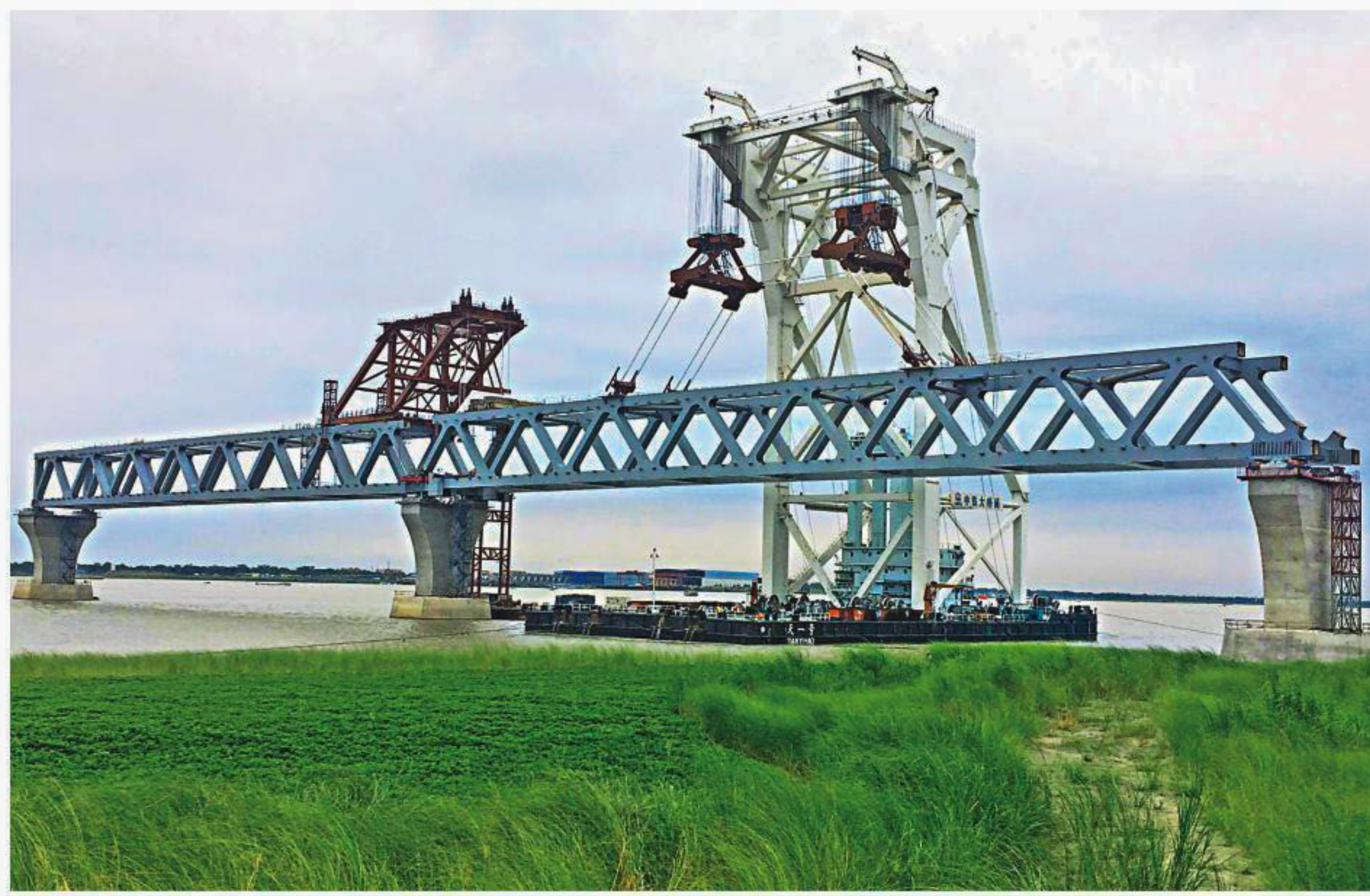
The 13th span of Padma bridge was installed on May 25. Upon assuming office, Finance Minister AHM Mustafa Kamal had announced that speedy implementation of mega infrastructure projects was his topmost priority.
