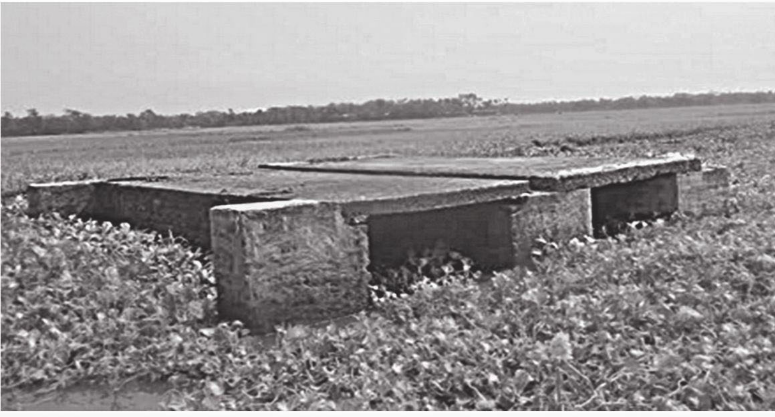
Built five years ago, this bridge on Pukuria Beel area of Sunampur-Surikhal road beside Kawadighi Haor in Rajnagar upazila of Moulvibazar has remained useless as the authorities concerned are yet to build approach roads on both sides. PHOTO: MINTU DESHWARA
