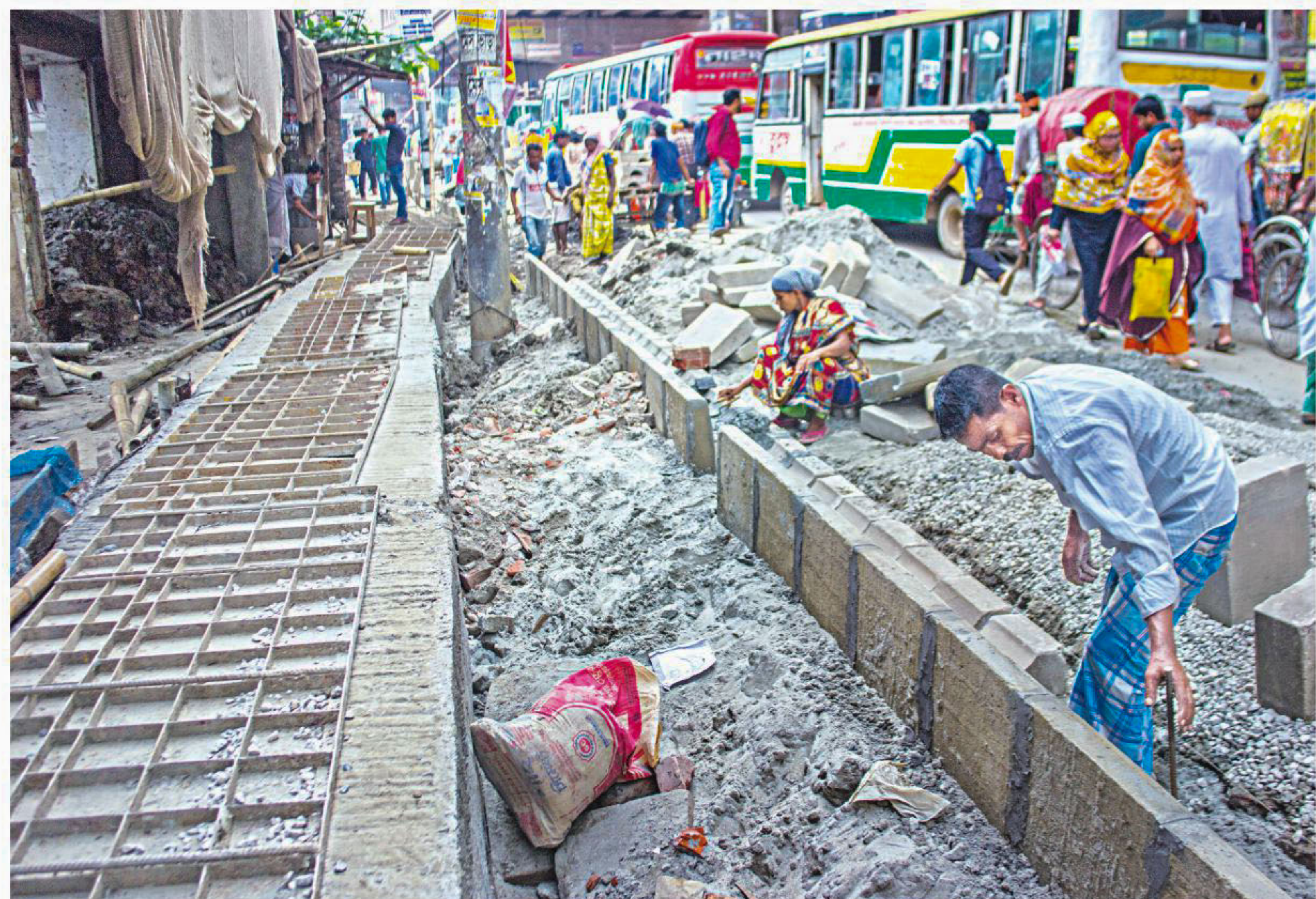
Pedestrians are forced onto the street as a pavement along the DIT Road is being rebuilt in the city's Malibagh. Construction materials are piled up on the road, causing tailbacks in the area. The photo was taken on Monday.
