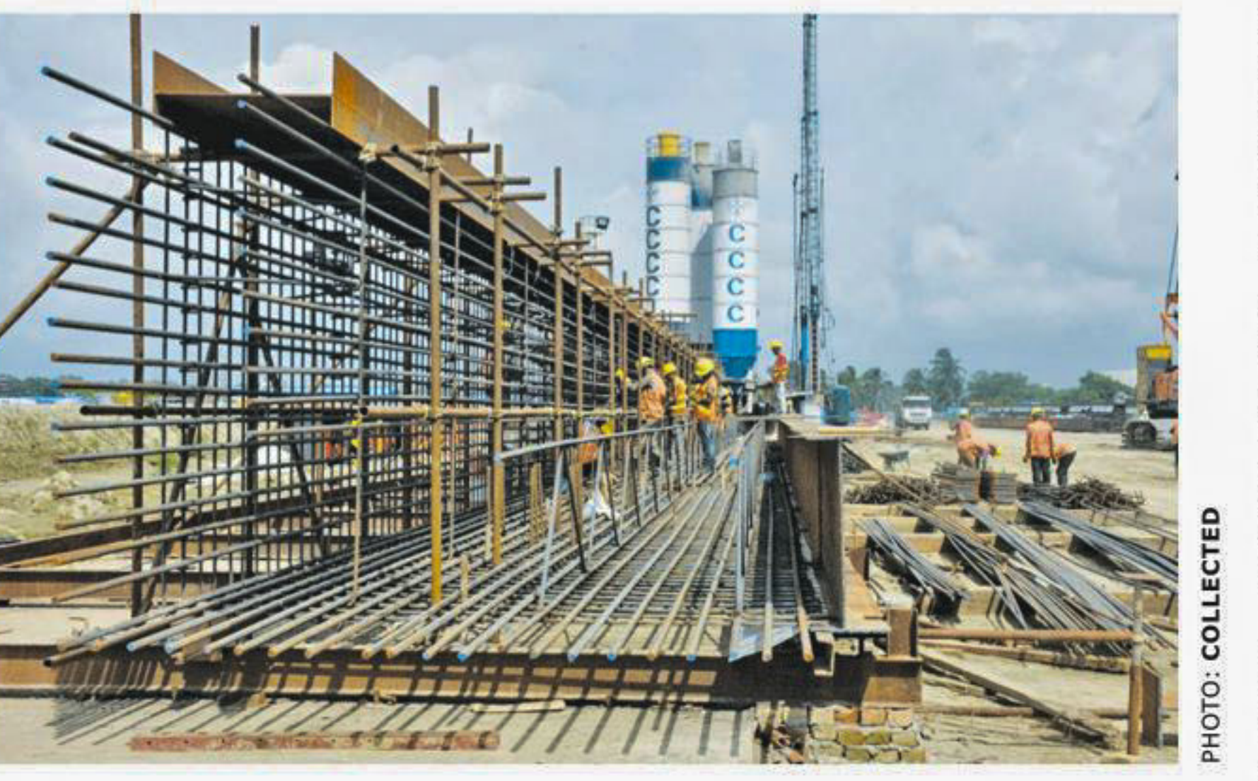
Construction work going on for the Karnaphuli tunnel which is a BRI project.
