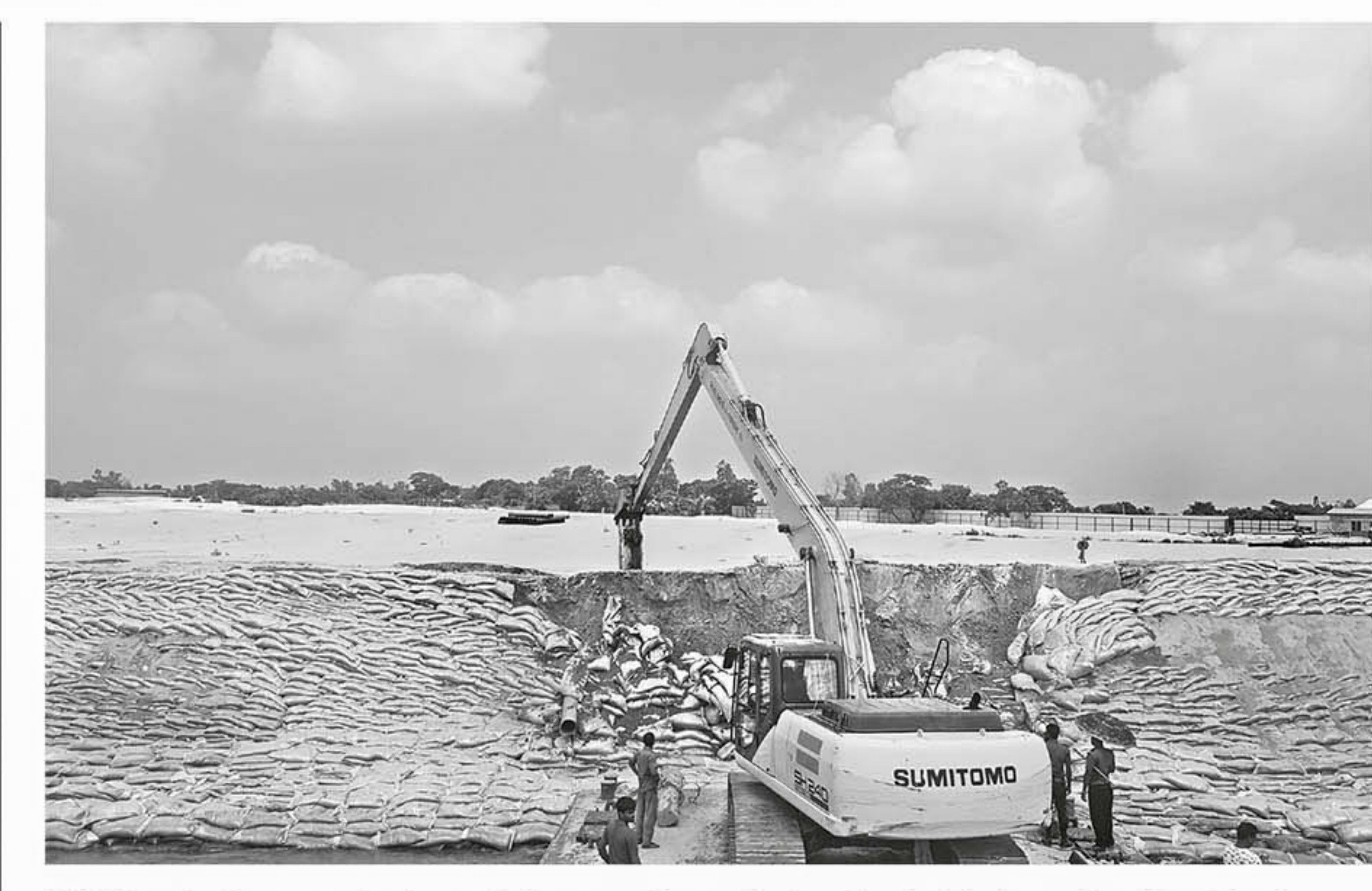
BIWTA knocks down an embankment, built encroaching on Meghna river, in Gajaria upazila of Munshiganj yesterday afternoon. As part of an ongoing drive to free the river, the officials also dismantled 30 illegal structures and cleared illegally piled sand and stones from the river, which were later auctioned off.
