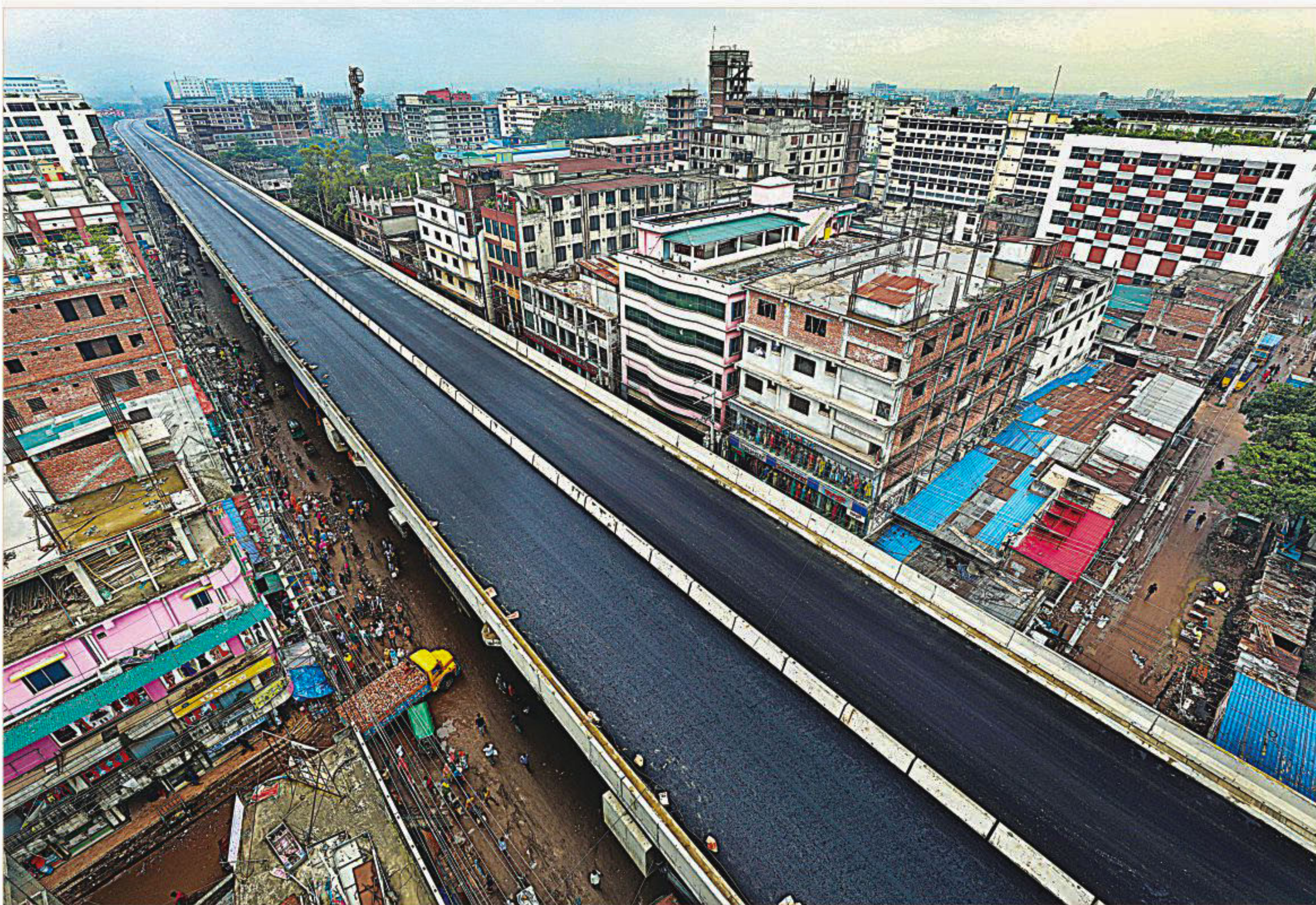
The construction of Konabari flyover on Dhaka-Tangail highway in Gazipur is complete. Prime Minister Sheikh Hasina will open the flyover to traffic today. The photo was taken yesterday.
