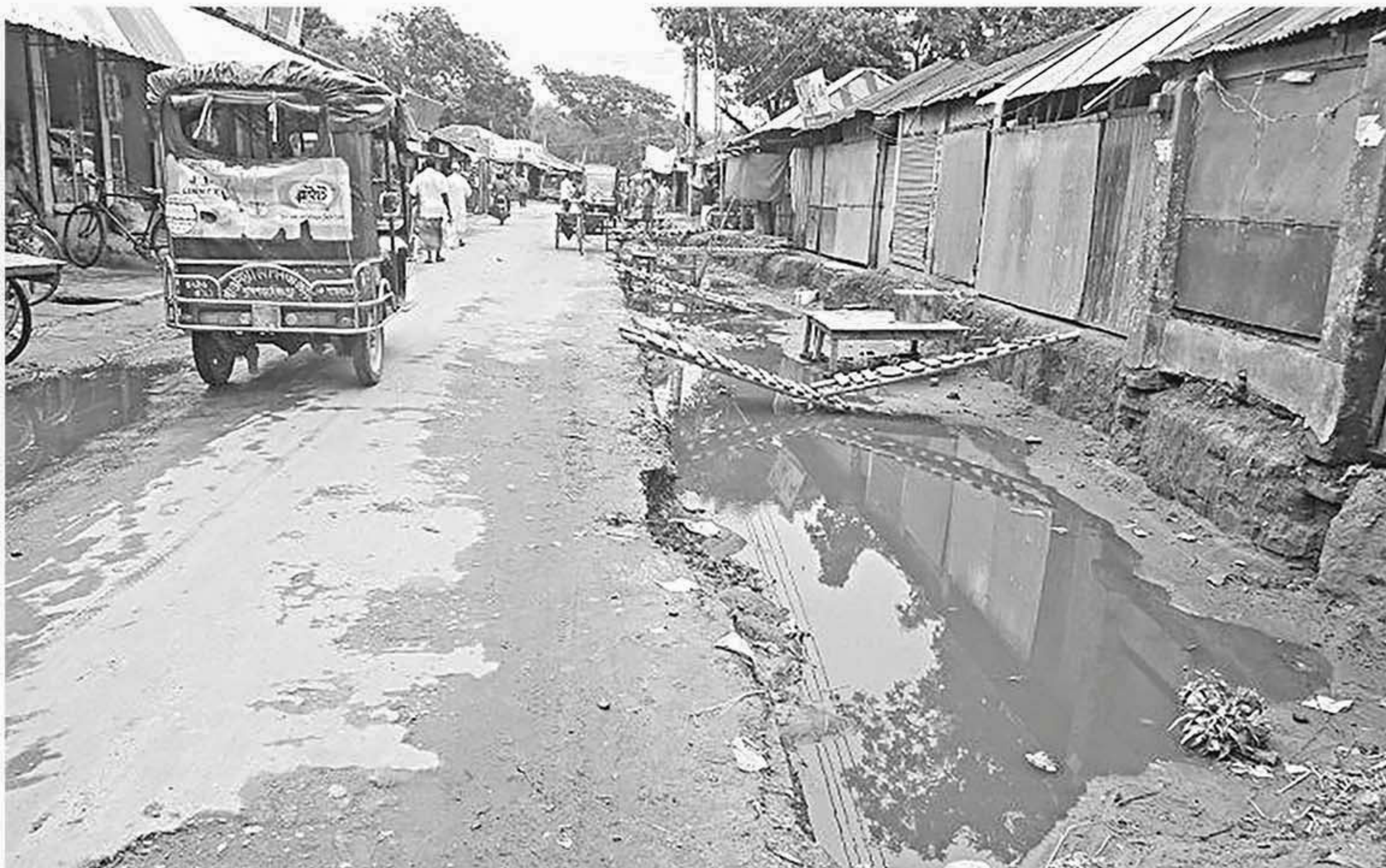
A ditch, dug to widen Birganj-Khansama-Darwani road three months ago, is yet to be filled at Darwani Bazar in Nilphamari Sadar upazila, causing immense sufferings to passengers.
