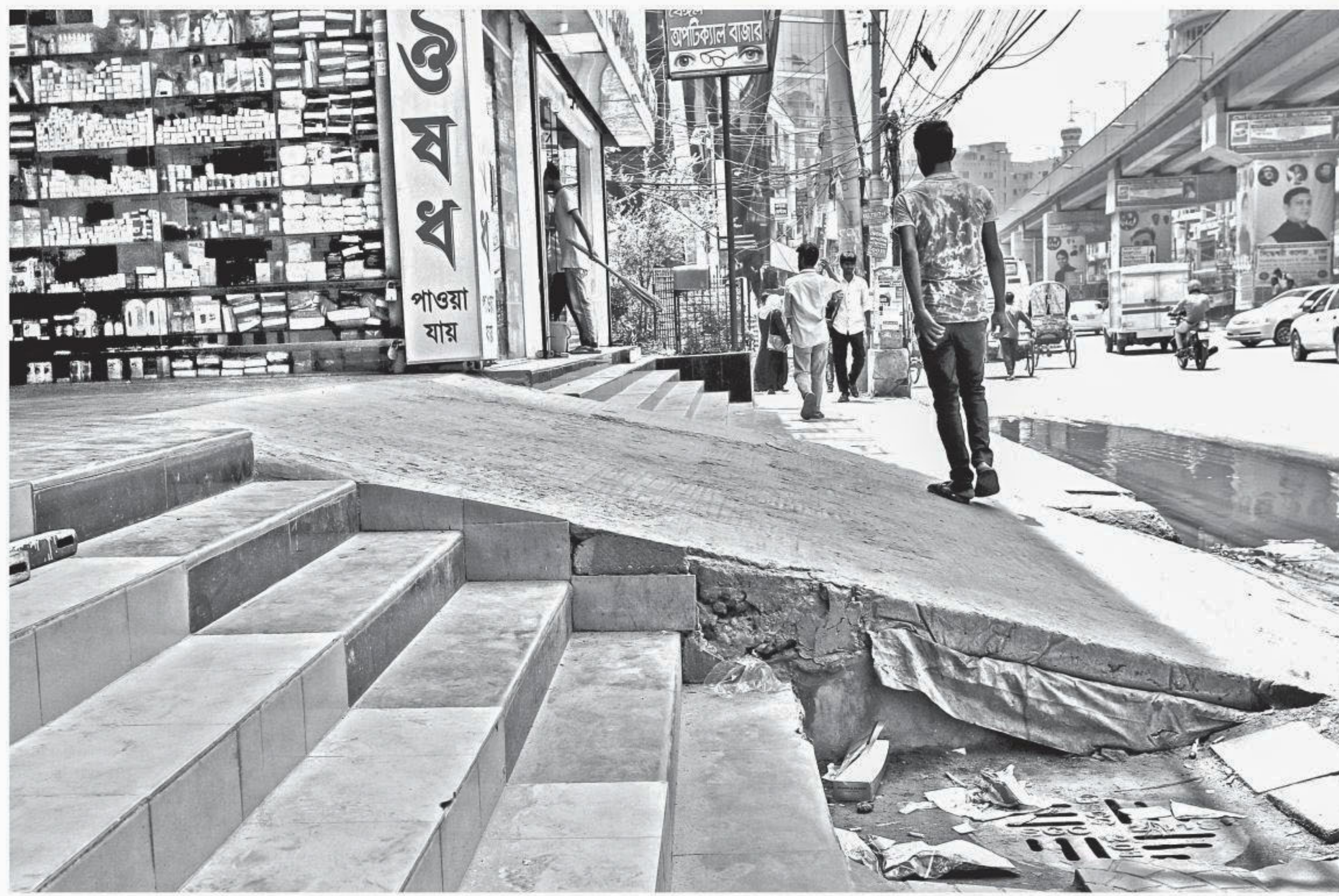
WHOSE FOOTPATH IS IT ANYWAY? An access ramp has been built occupying a part of this footpath to facilitate exit and entry of cars in Dhaka's Siddheshwari. City corporation authorities had demolished such illegal extensions in the area few months ago, but several building owners have rebuilt these, in a blatant disservice to pedestrians.
