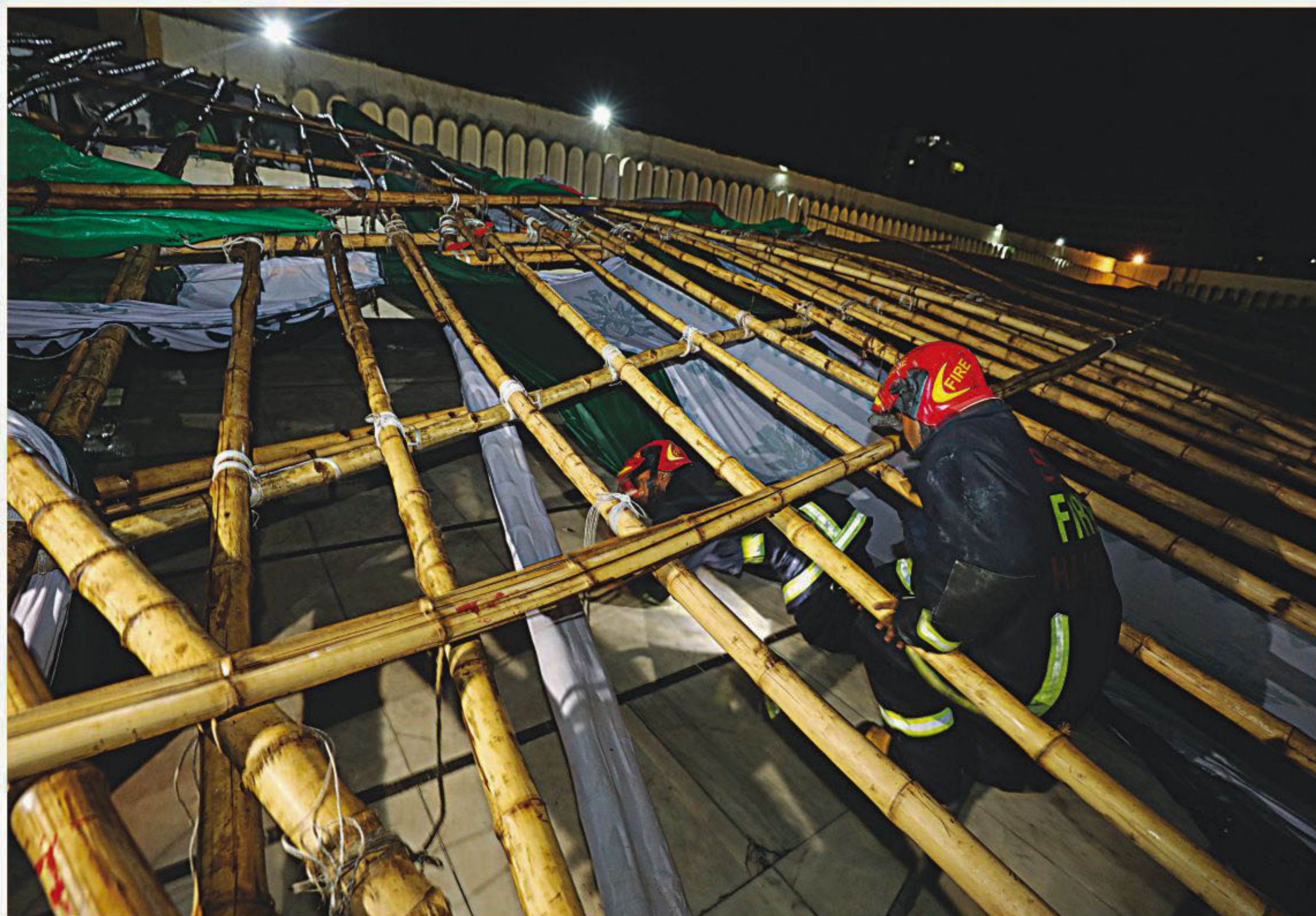
Firemen search for people trapped under the pandal at Baitul Mukarram national mosque in the capital yesterday. The pandal collapsed during a storm in the evening. The accident left one person dead and around 22 others injured.
