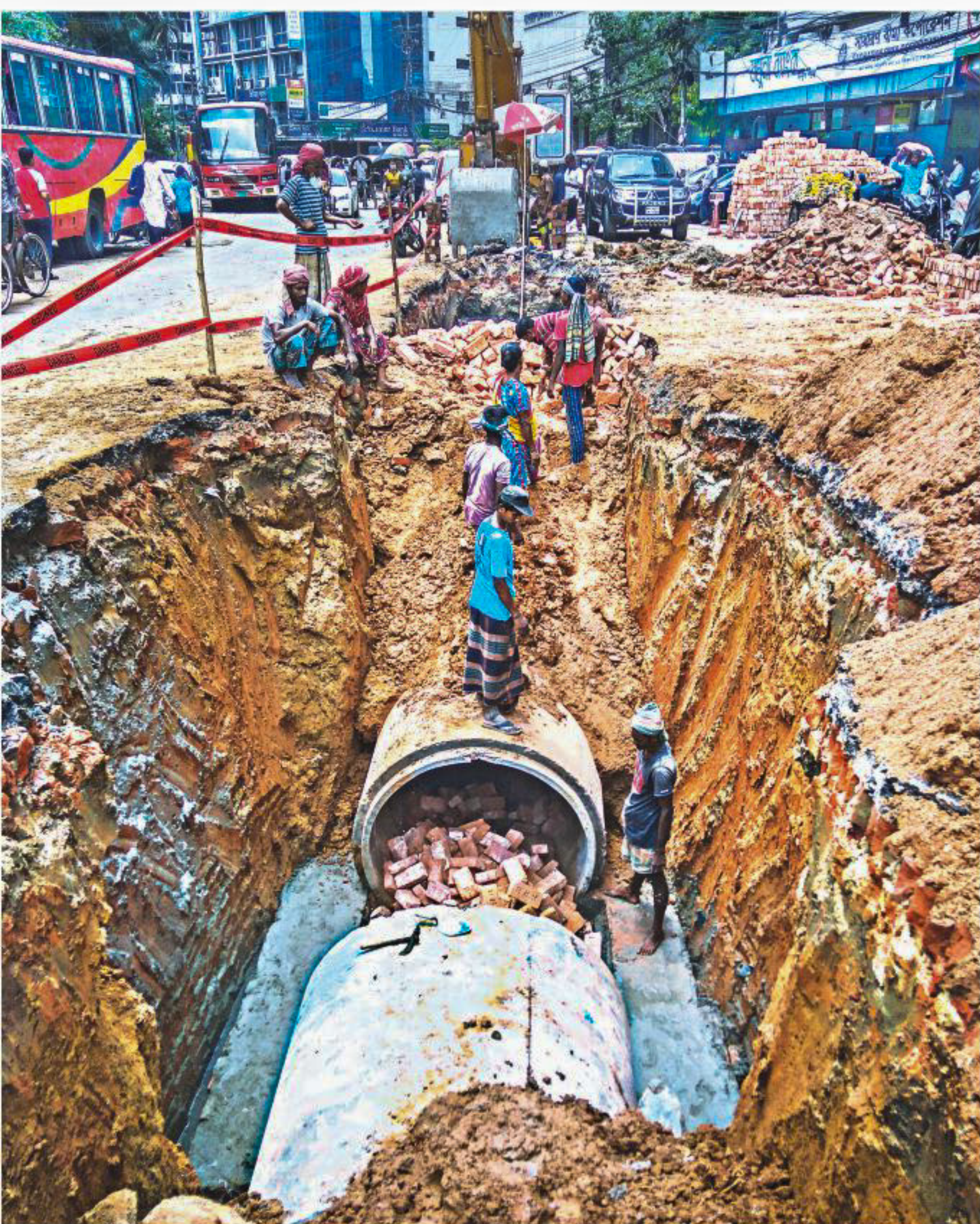
City corporation workers busy setting up pipes in a trench dug up on a road in Motijheel's Dilkusha area. Though the work has been continuing for a while as part of a drainage development project, DSCC apparently forgot to put up safety barriers other than a flimsy cautionary tape. Be it day or night, this road is used by pedestrians and vehicles alike.
