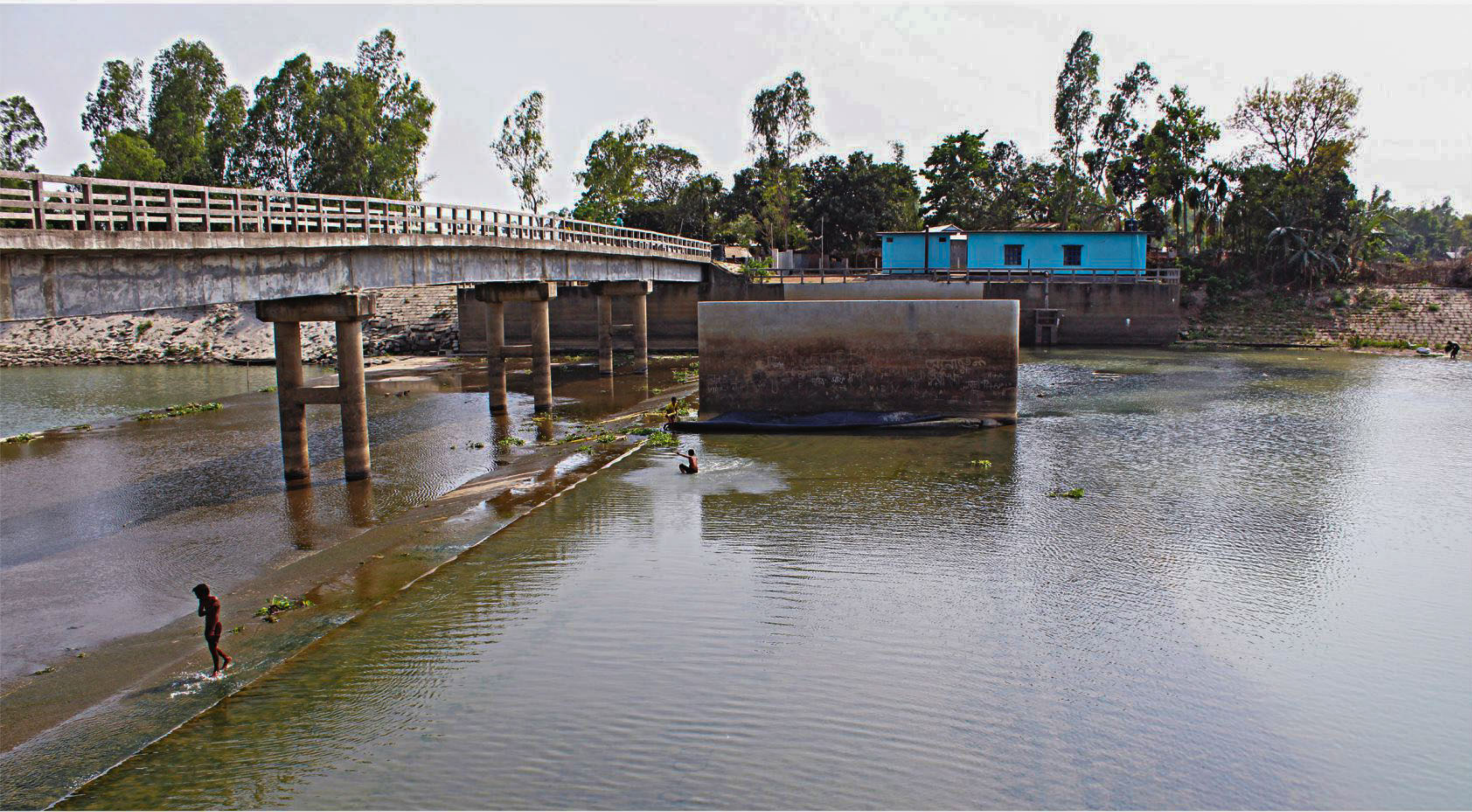
The inflatable rubber dam constructed at the cost of more than Tk 15 crore lies useless due to shrinking flow of the river.
