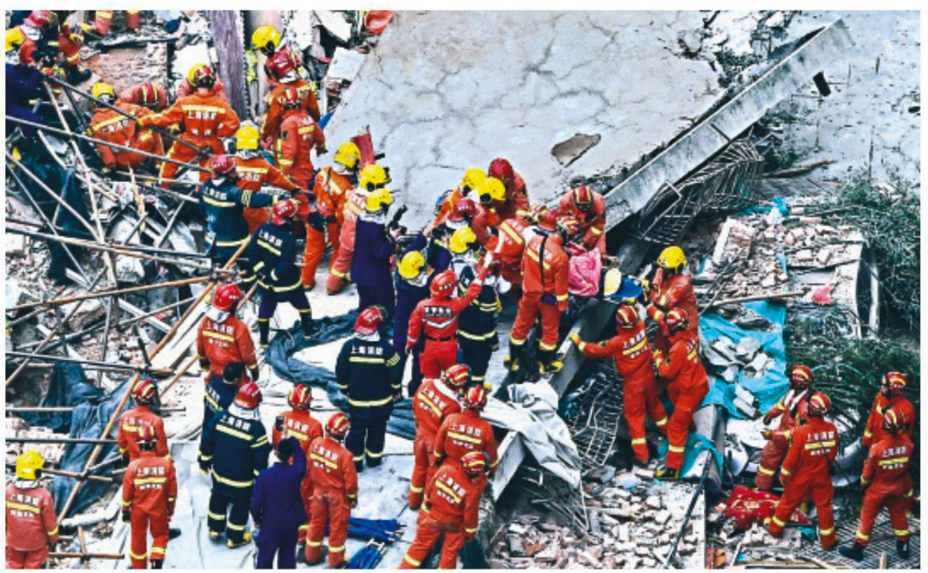
Members of a rescue team carry out a victim from a collapsed building in Shanghai, yesterday. At least seven people were killed yesterday when the roof of a Shanghai commercial building caved in upon construction workers who were renovating it, the city government said. 21 people had been pulled out of the debris and rushed to hospital.
