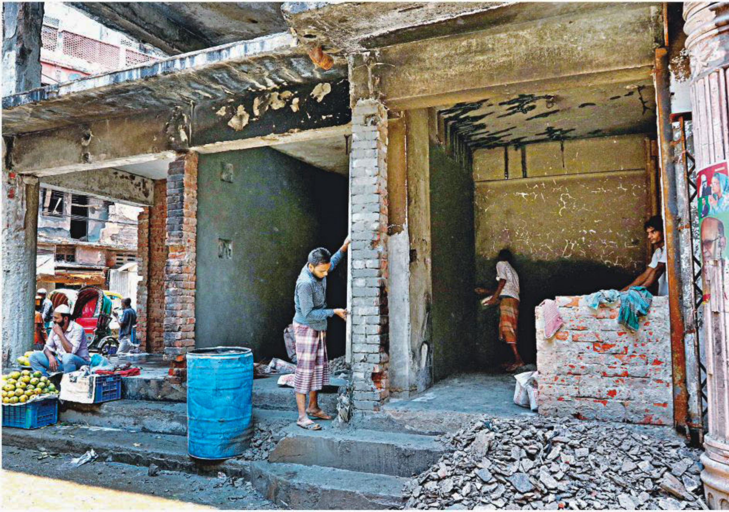
Shops on the ground floor of Wahed Mansion, ground zero of the Chawkbazar inferno, is being mended for reopening even though the building itself is at risk. The fire had left 70 dead and scores injured on February 20.
