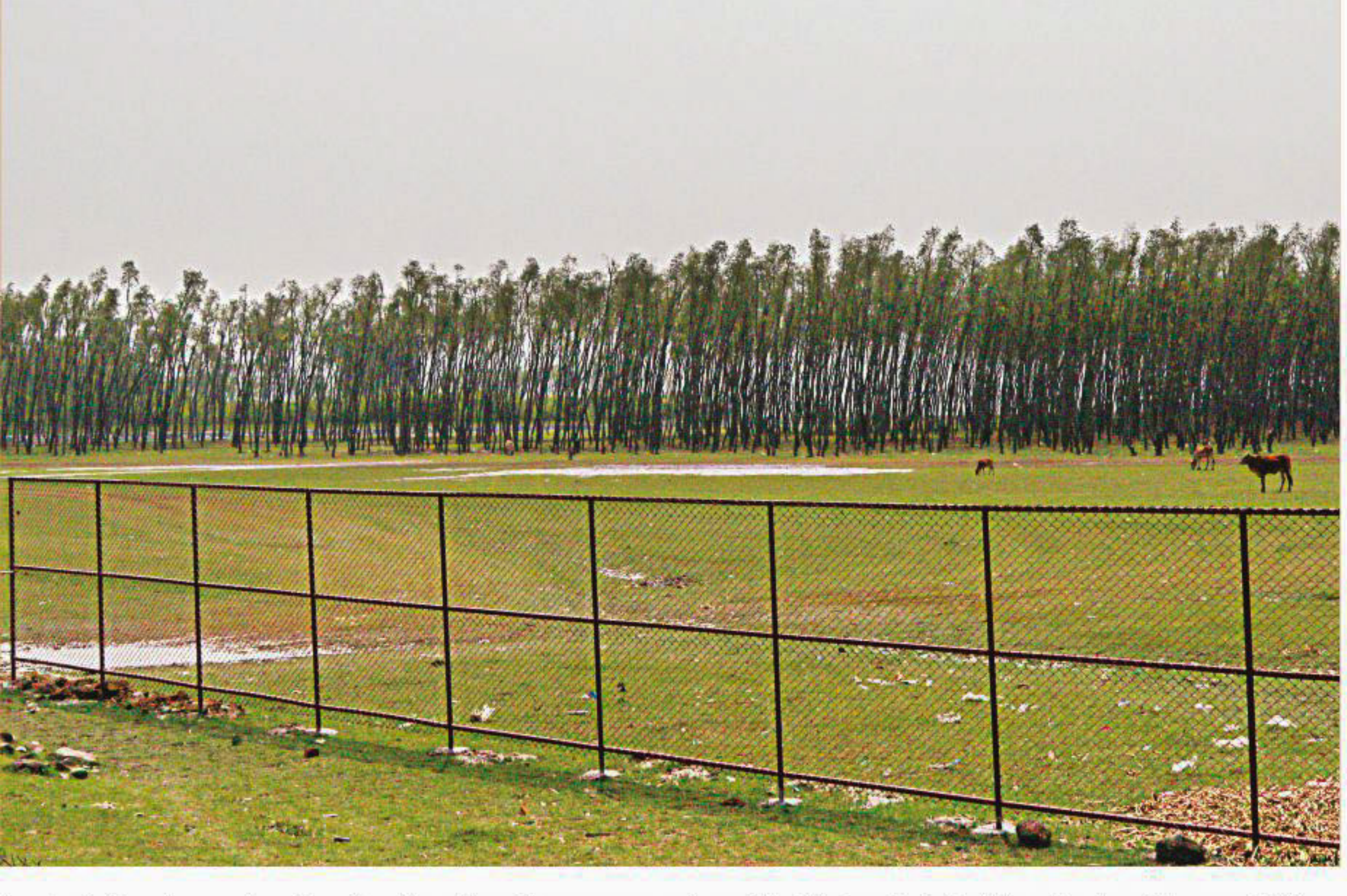
A private firm has put up iron fencing along the mangrove forest in Sitakunda to build a ship-breaking yard. The company took a lease on 7.1 acres of the forest land from the district administration last year. The photo was taken in Abdullah Ghata area last month. PHOTO: RAJIB RAIHAN
