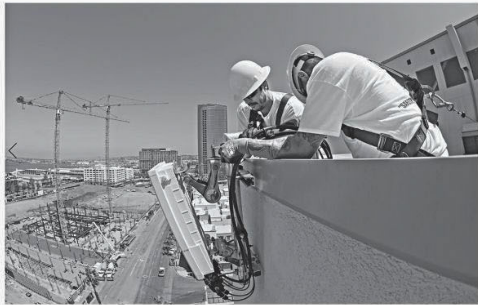
Telecommunications workers install a new 5G antenna system for AT&T's 5G wireless network in California.
