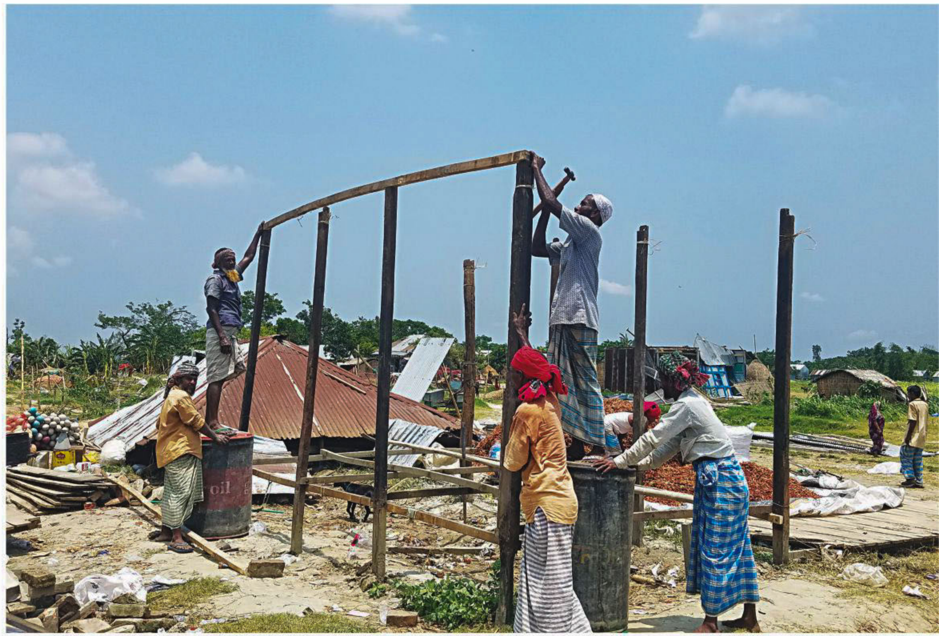
Workers construct a house in Chandpur's Rajrajeshwar union in the sadar upazila yesterday. When Cyclone Fani struck Bangladesh, it obliterated over 100 houses in the area and damaged many more. Around 14 people also died in different parts of the country during the cyclonic storm.
