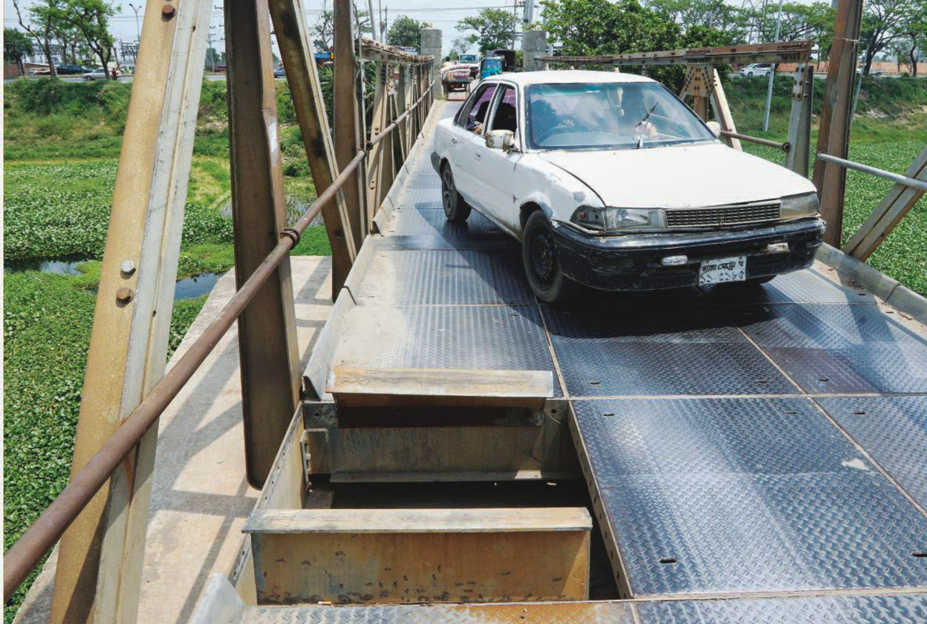
The authorities removed parts of the metal floor of a Bailey bridge on the Savar-Bhakuta road and raised the edges of the gaping hole so that heavy vehicles cannot use the bridge not meant for them. The authorities, however, created a death trap as anyone could fall into the canal below. PHOTO: PALASH KHAN
