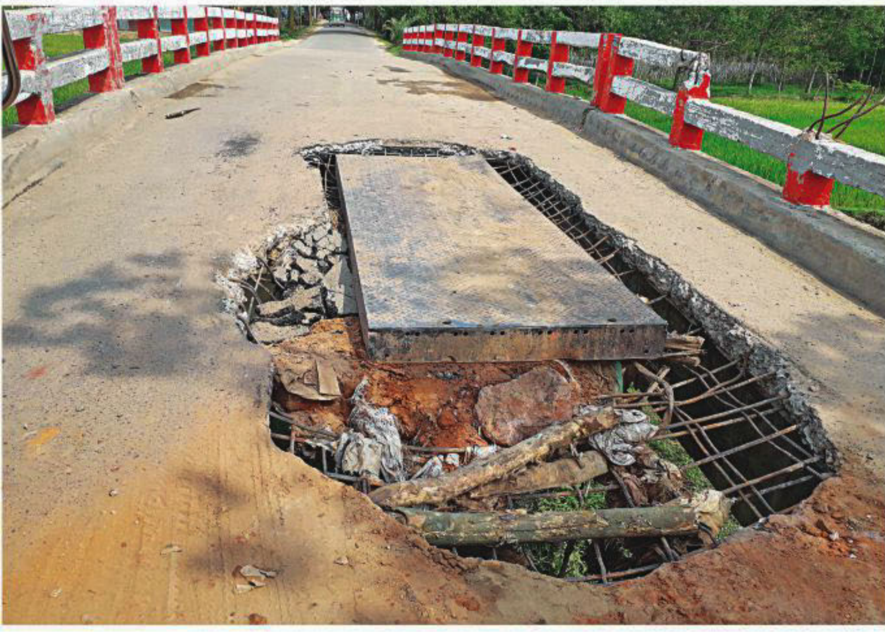
A large chunk of this bridge in Bijoy Nagar of Brahmanbaria broke and fell into the Kaikkayachora canal beneath. A steel plate was later placed there as a stop-gap solution but with iron rods sticking out, it remains unsafe as before.
