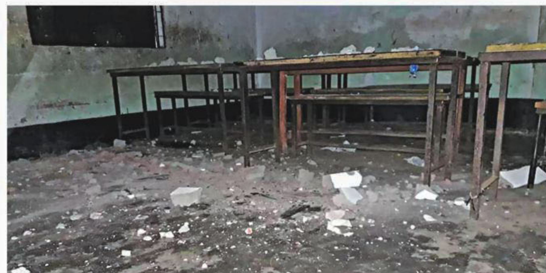
Spalling of concrete from the soffit of the slab of a school building.
